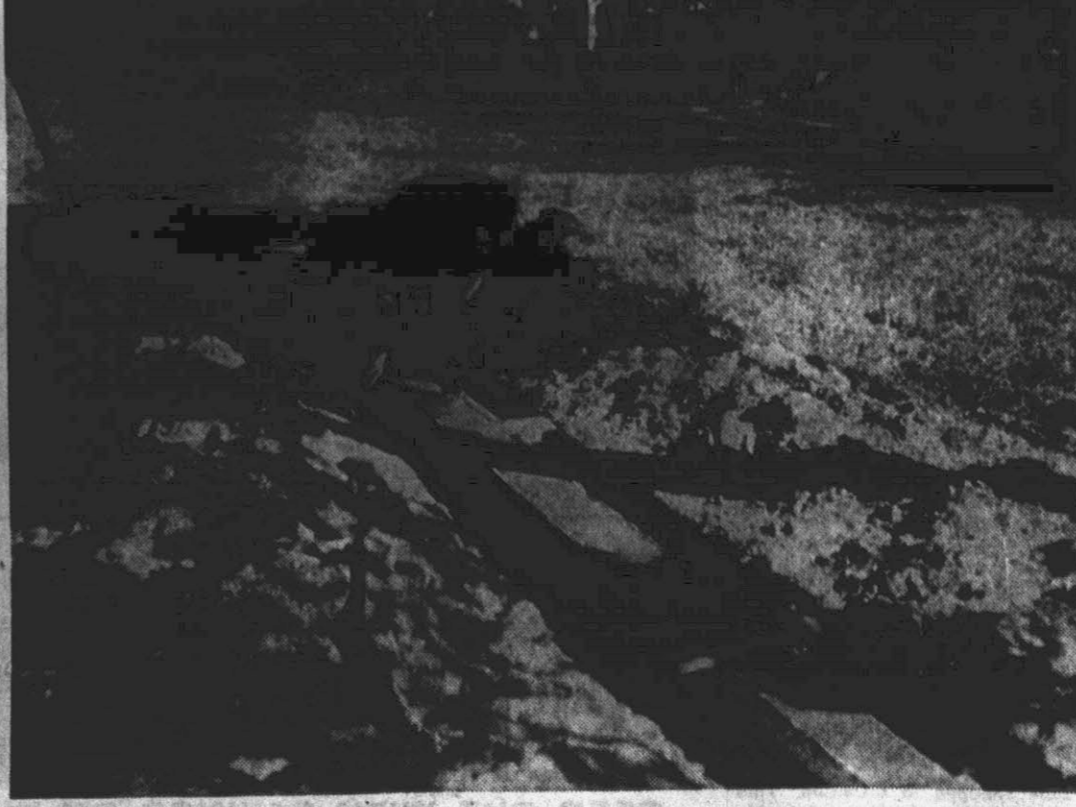
Workmen put the finishing touches on a curb for a drive which will pass behind Sheppard Memorial Library. The drive leads to an area which will be used by the Bookmobile. It is to be paved at a later date. Reflector photo by Alvin Taylor.
