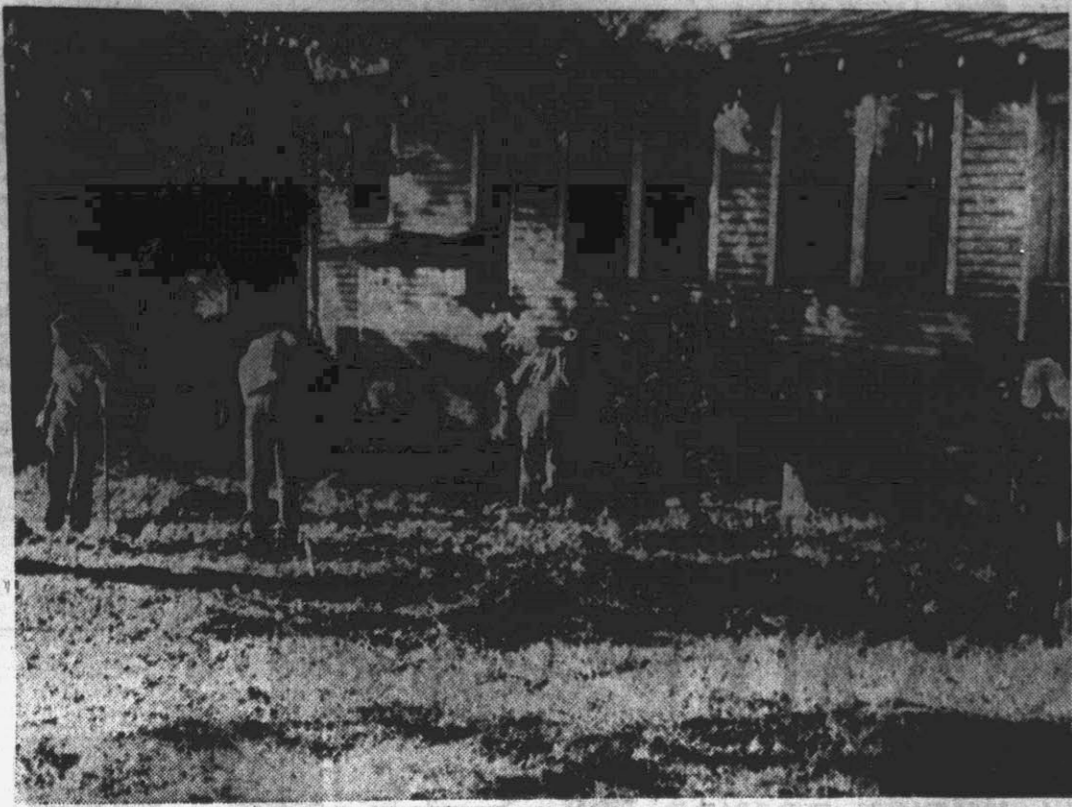
Workmen are shown here as they dig a trench preparatory to the installation of curbing for a drive on the Sheppard Memorial Library grounds. This is another step in the plans of the city and the local Garden Club for beautification of the library lawn. When the drive is cut, the lawn will be regraded and seeded by the city and new trees and shrubs will be planted by the Garden Club. (Reflector photo by Edwina Haymes).
