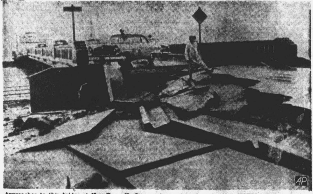
Approaches to this bridge at New Bern, N. C., were battered to pieces by high waves whipped by hurricane Ione. Numerous motor vehicles were marooned in the vicinity of the bridge. Four persons were killed by the hurricane in the New Bern-Morehead City area and property damage ran into the millions of dollars. (AP Wirephoto)
