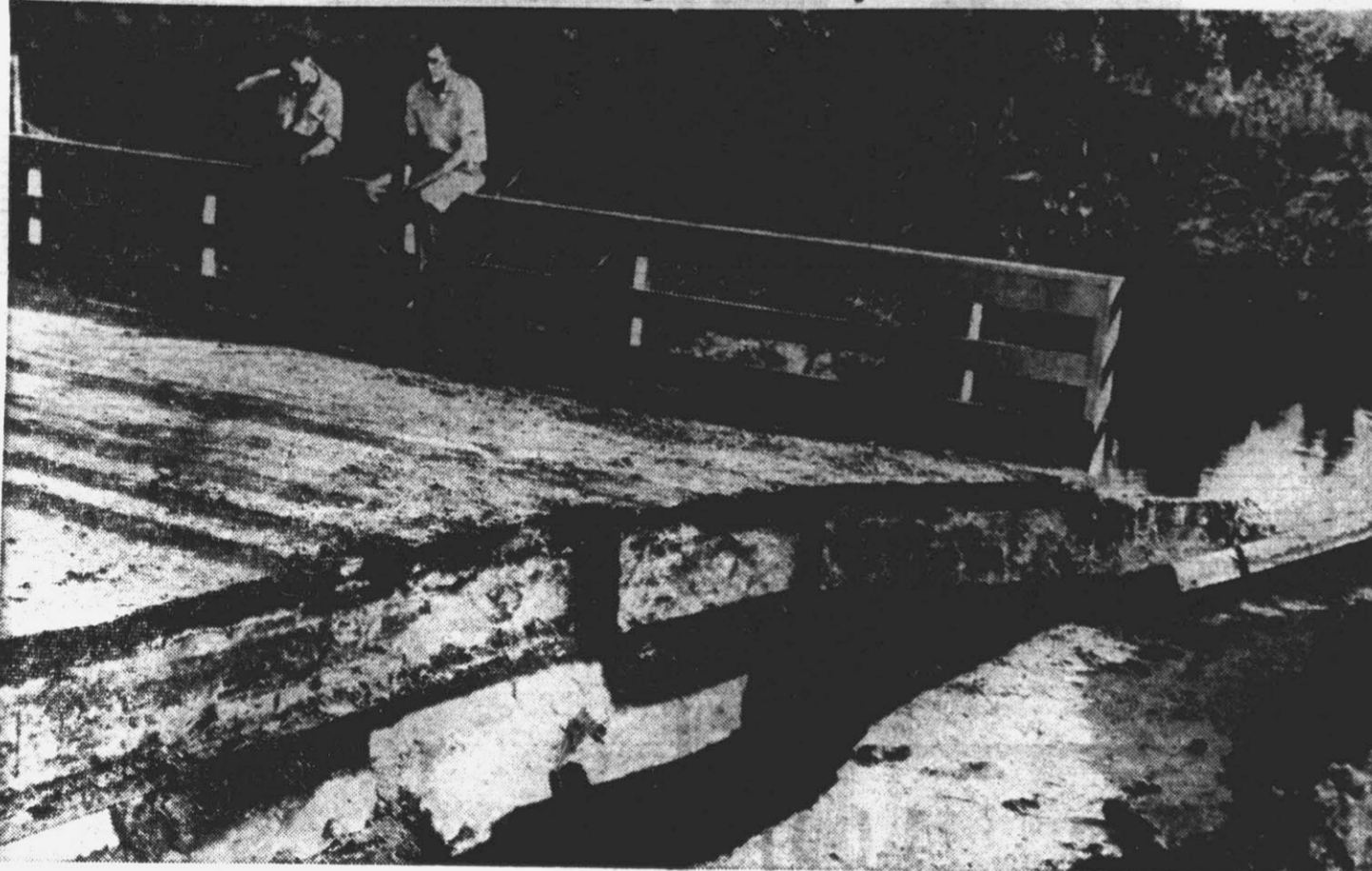
Washouts have been a big problem to the highway department since Hurricane Ione hit the Eastern Carolina section. The old Stantonsburg road between Greenville and Farmville was closed after the road way leading to the above bridge washed away. Highway crews have been busy since the storm striking the damaged road ways. (Reflector Photo by Alvin Taylor)
