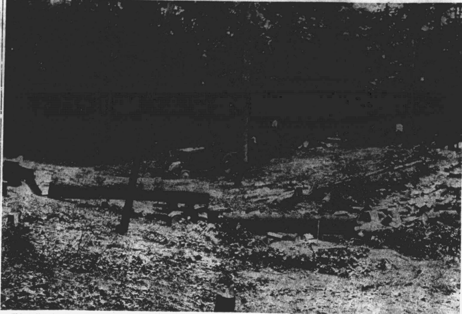
This is the site of the new outdoor theatre which is being constructed on the western edge of the East Carolina College campus. Work on the theatre has already begun. The sum of $10,000 was given by Mrs. Rosa M. Flanagan and the theatre will be a memorial to her husband, the late E. G. Flanagan. (Reflector Staff Photo).
