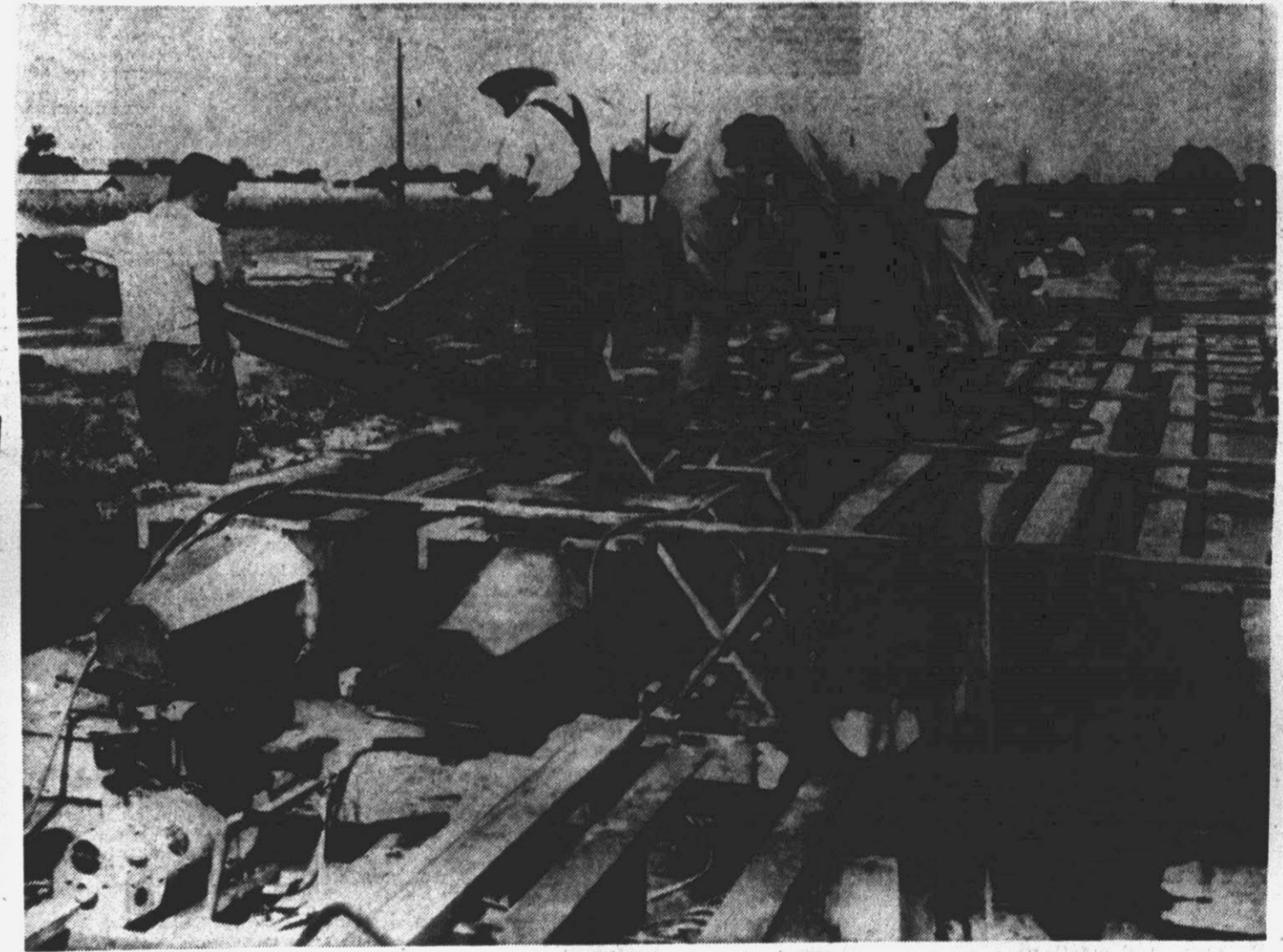
Workmen are pictured above as they pour concrete into the steel molds to form the pilings which will support the new highway bridge over the Tar River and two overflow bridges. Some 60 such pilings each 52 feet in length will be needed to do the job.
