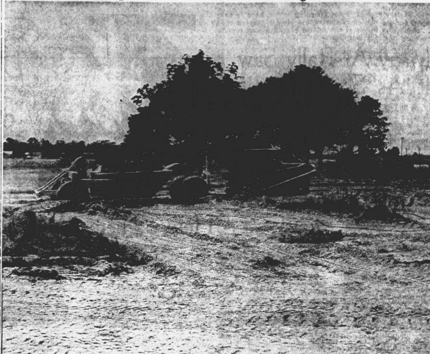
Leveling of land for the new Greenville high school is now under way. A big drag pan is shown above as it moves about the school site on Elm St. The senior high school building is expected to be completed by late fall of 1956 or by January 1, 1957 at the latest, according to school authorities. Cost of the building is to be $822,855. (Reflector Photo by Alvin Taylor.)
