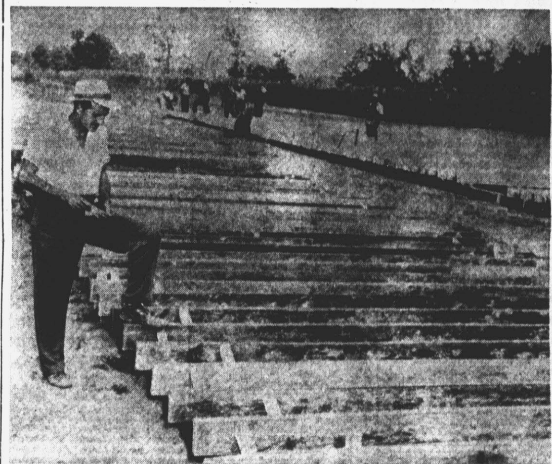
Superintendent of Bridge Work Gordon Parker is shown above as he looks over the forms on which concrete piers will be poured for the new Tar River bridge. Some 60 piers are to be sunk to support the main bridge. In addition 60 more will be needed for two overflow bridges.
