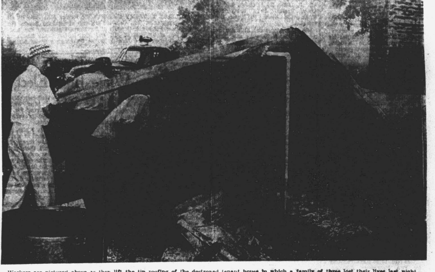
Workers are pictured above as they lift the tin roofing of the destroyed tenant house in which a family of three lost their lives last night. The body of a 12-year-old boy was found at the spot where the volunteer workmen are probing in the above photo. In the background can be seen the Ayden fire truck which was called to the scene to cool the smoldering wreckage so the bodies could be removed.
