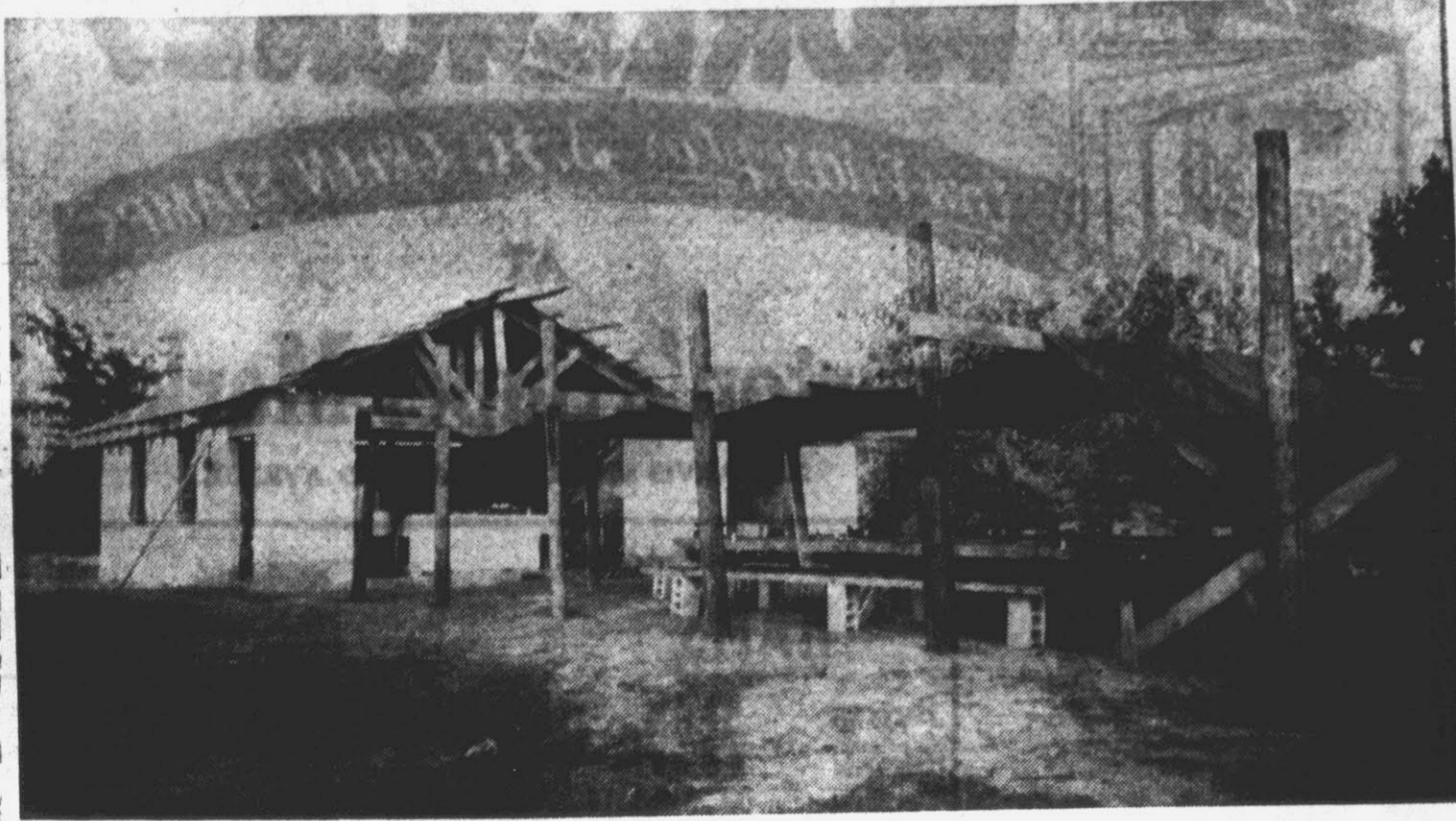
Pictured above is the concrete block dining hall which is being constructed by volunteer labor at the new Negro boy scout camp located on Kerr Lake three miles west of Drewery, N. C. The building is being constructed under the direction of Herman R. Foust of the C. M. Eppes High School faculty.
