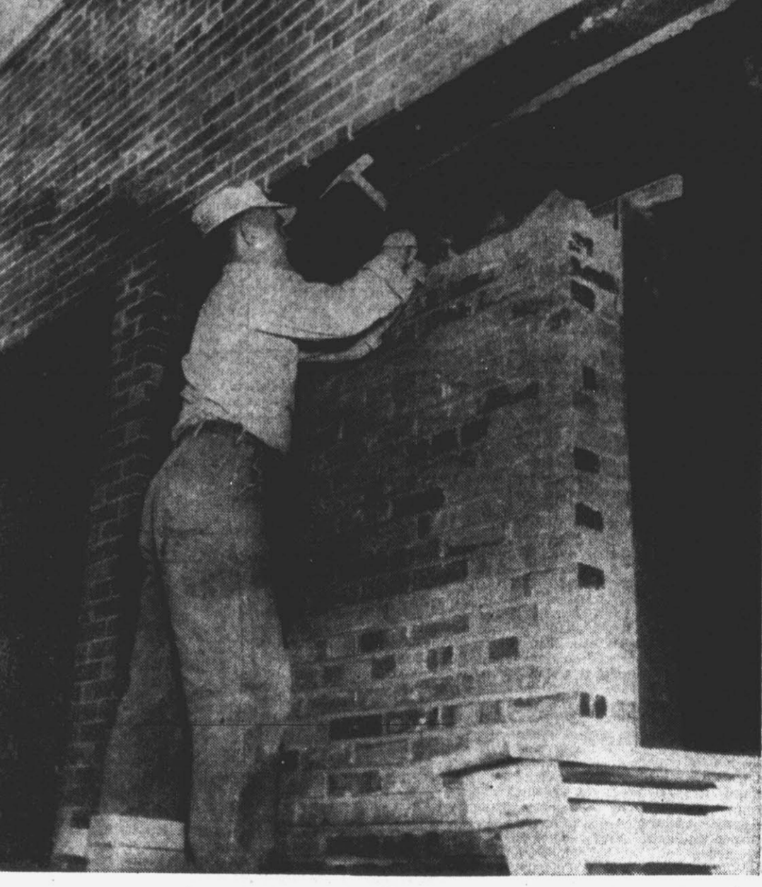
REPAIRS IN PROGRESS—Workers at the National Guard Armory here are well on their way to completing the installation of new overhead doors to replace wooden ones formerly in use. The work pictured above is part of a renovation program that includes the installing of fans, improvement of the firing range and kitchen. (Reflector Photo by Bob Hilldrup.)
