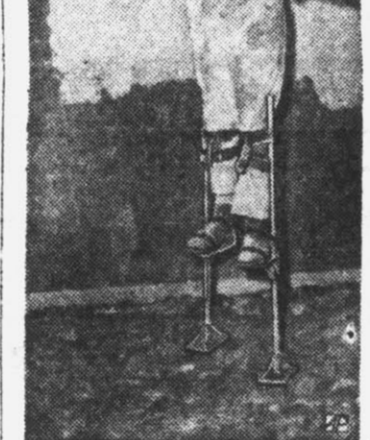
AP Newsfeatures EASY WAY to plaster a ceiling: wear aluminum stilts. They save workers more time and trouble than using long scaffolding.
