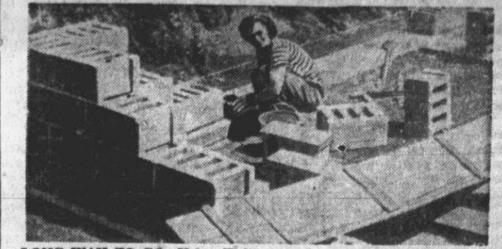
LONG WAY TO GO—Helen Welty puts down the first cinder blocks at home-to-be in Fairborn, Ohio. They used mail-order house plans.
