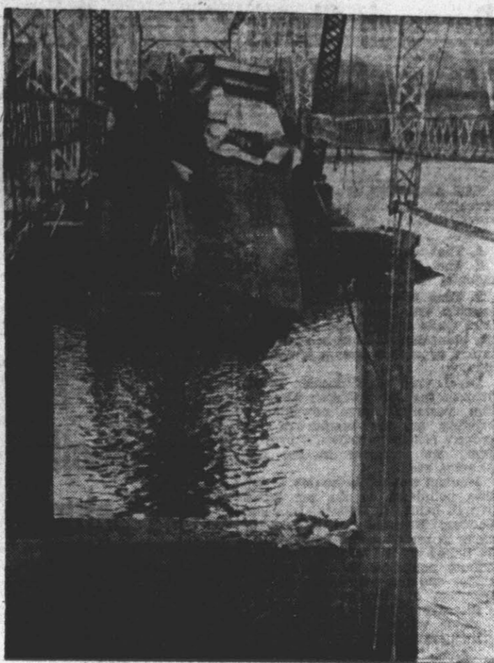
SAVED BY INCHES — The driver of the tractor-trailer rig shown here is a lucky man. Virgil Phillips of Birmingham, Ala., suffered only fright when a 100-foot section of the 507-foot span over the Elk River, north of Decatur, Ala., collapsed as the heavy truck passed over it. (AP Wirephoto).
