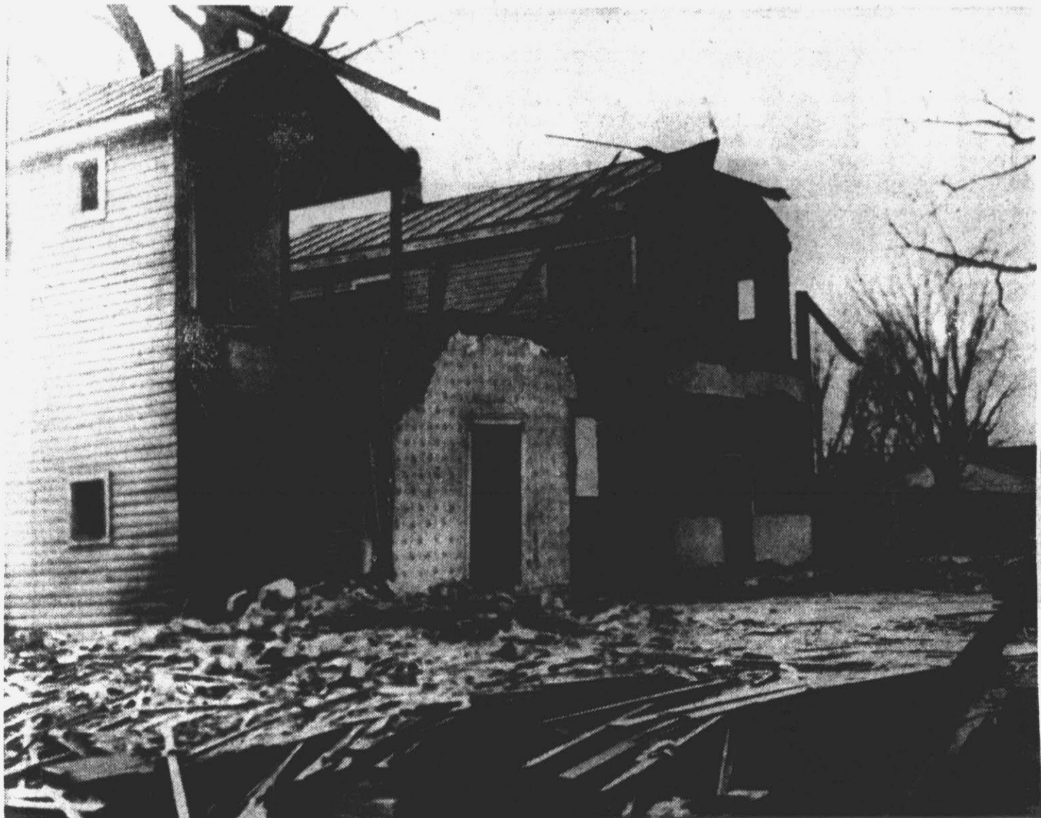
This is not a civil defense scene or bombed-out European or Asian Building. It is the old Horton Hotel in Farmville which was being torn down by board this week, because of old age, decay, and the mounting cost of keeping an ancient building in repair. The picture above is a view of the back portion of the building, in a nest of shambles. (Reflector Photo by Alvin Taylor).
