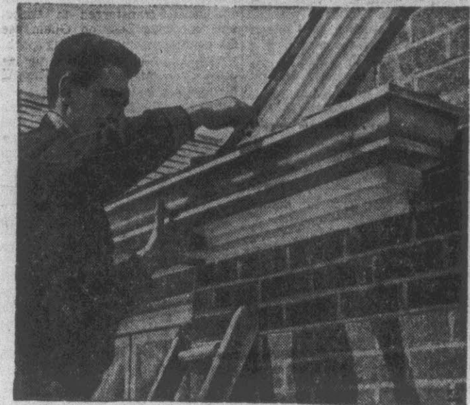
DON'T MIX your metals on the roof. One metal will eat the other away. This man is using the same metal for hangers and supports as the eaves trough metal.
