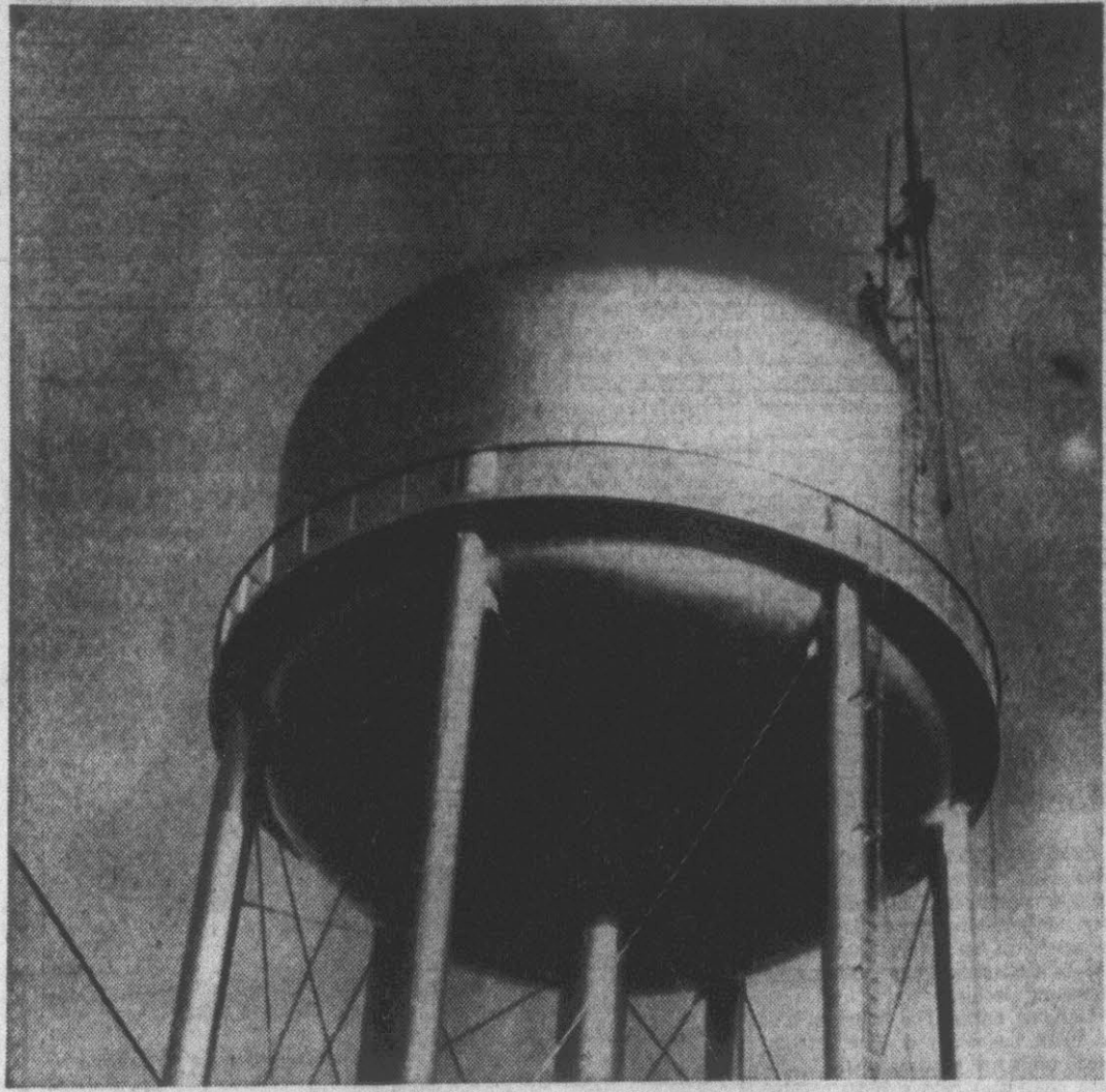
Workmen are pictured above atop the water tower on North Greene Street as they install the base for an antenna which will be used for transmission by the Greenville Utilities new two-way radio. Initially six of the utilities trucks will be outfitted with radio units. (Reflector Photo by Alvin Taylor).
