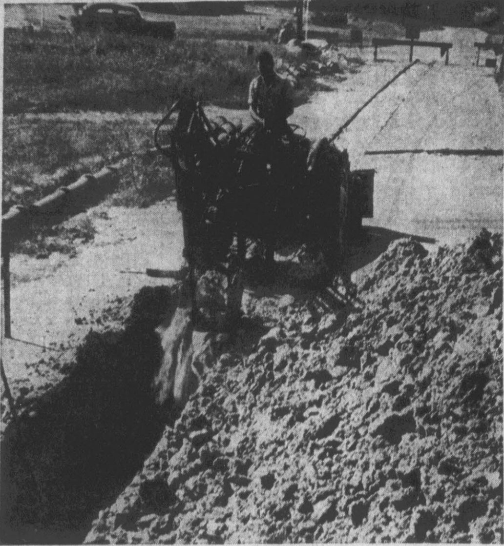
LAYING SEWER LINE FOR ELMHURST — Greenville Utilities workers are shown digging ditches for installation of sewer lines for the Elmhurst section. The lines will serve the new school now under construction as well as homes in that section. It ties in with the Forbes Run outfall line. (Reflector Photo by Alvin Taylor).
