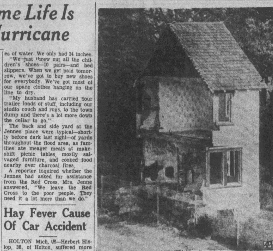
SOUTHERN EXPOSURE—Most of the home of Louis Gitlin was in the path of the Delaware River Turnpike extension through Willow Grove, Pa., linking the Pennsylvania and New Jersey turnpikes—so that part of the house had to come down. The part that was on ground not taken over by the turnpike authority doesn't concern highway engineers—so, they left that part standing. Gitlin and three brothers have battled the turnpike since the extension was started, at one time holding off the workmen with shotguns. They now are engaged in litigation over damages the authority will pay for their properties. (AP Wirephoto)
