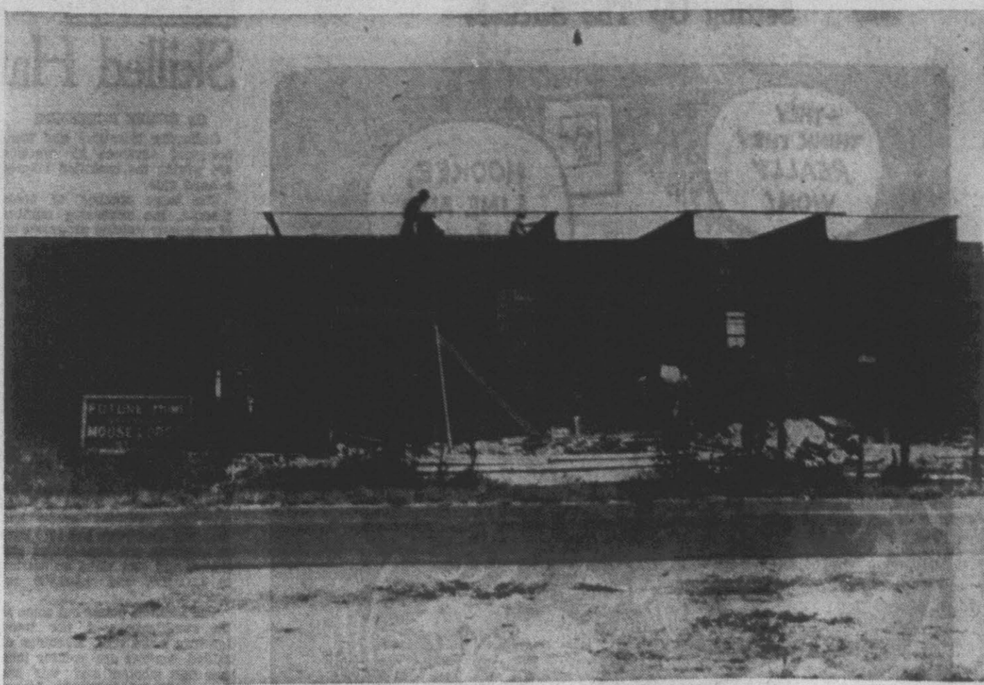
SEVENTY PERCENT COMPLETE —The new Moose Lodge, shown here, is about 70 percent completed. Moose members hope to move into the new modern, air-conditioned building that includes a 600 seat auditorium in the latter part of November or early December. The building, which contains about 11,000 square feet of floor space, will also contain dining facilities, reading room, TV room and a game room. The Moose membership now exceeds 400 and it is hoped to have 600 members by the time the new Lodge is occupied. (Reflector Photo by Bob Boyette)
