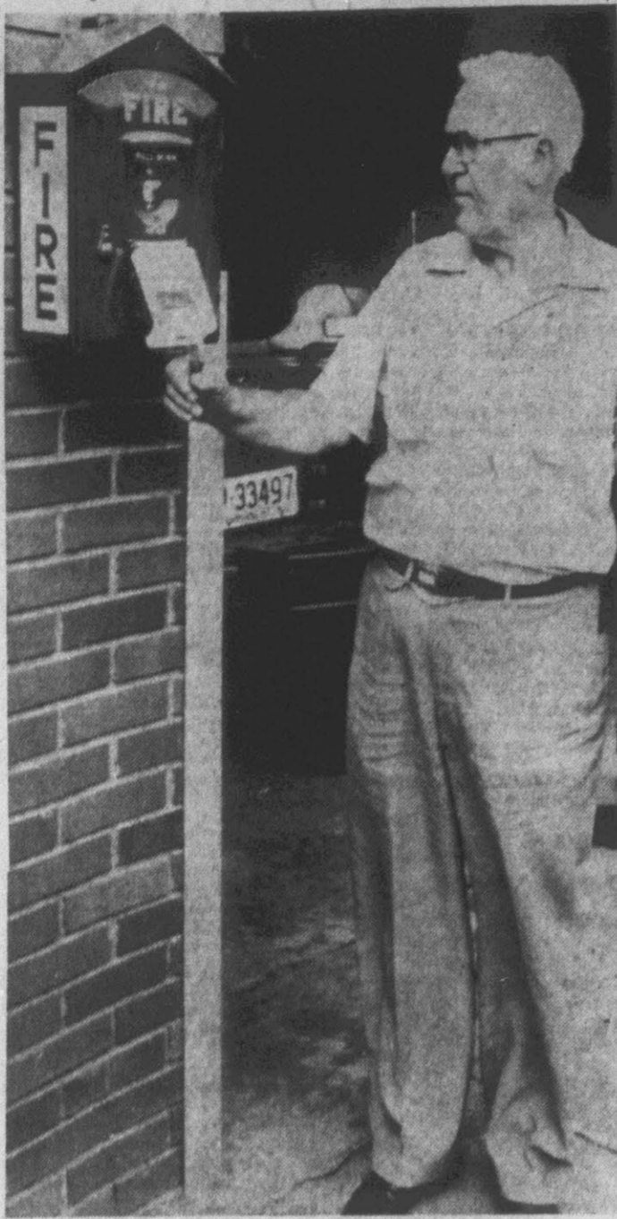
A. W. Sawyer, Superintendent of Ayden Utilities, is shown testing Ayden's first installed fire alarm box, which is placed in front of the fire station. Other boxes are being installed at various locations in the city. Upon completion of the installation of alarm boxes there will be approximately fifty. The town is very proud to have this improved convenience in turning in the fire alarm. (Photo by James W. Everett)
