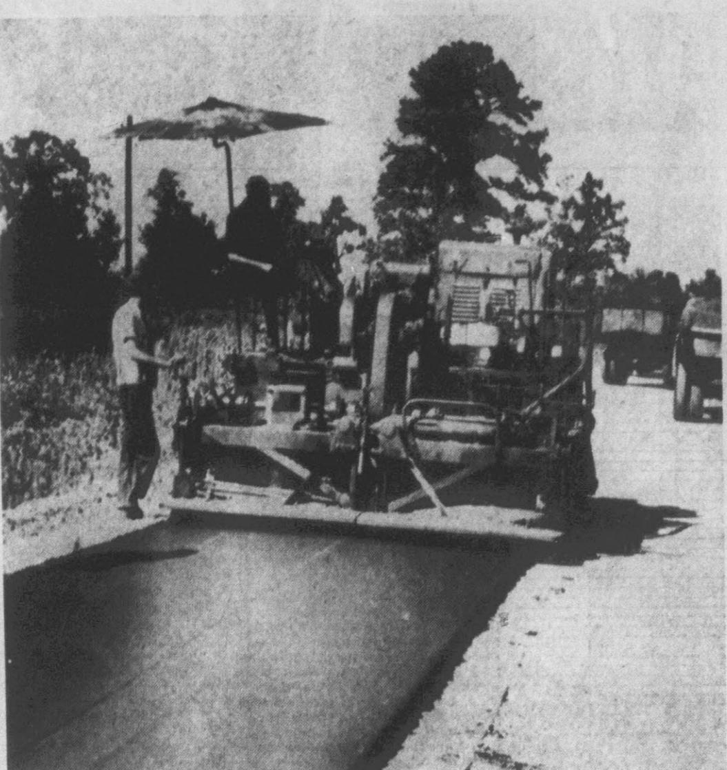
Workers are shown above as they pave the approaches to the new Tar River bridge at Grimesland which will probably be opened to traffic by the time school opens, according to the State Highway Commission. The bridge, constructed at a cost of $239,000, was begun on February 9, 1953. The old bridge west of the new river crossing is to be torn down.
