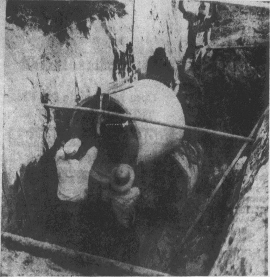
Workmen are shown installing storm drains in Hillsdale. The drains will drain the entire area of Hillsdale. The total length of all the pipes, which range from 12 inches to 26 inches, is 4,700 feet. During the project some of the streets will be regraded so there will be surface drainage to the catch basins. When the job is completed the streets will be "final grade" and ready for paving. Low bid on the project was held by White Construction Company at a cost of $31,509.50. (Reflector Photo by Alvin Taylor)
