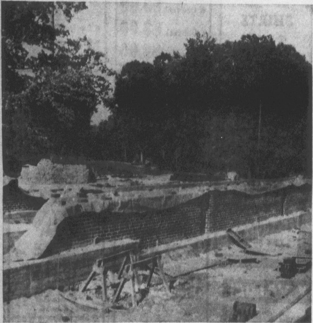
Pictured above is the new men's dormitory now under construction on the campus of East Carolina College. The new dorm is located just behind Slay Hall and faces Tenth Street. It will provide space for 310 students and is being constructed at a cost of $650,000. The new dormitory is to be named William B. Umstead Hall and expected completion date has been set for September 1, 1955. (Reflector Photo by Alvin Taylor)
