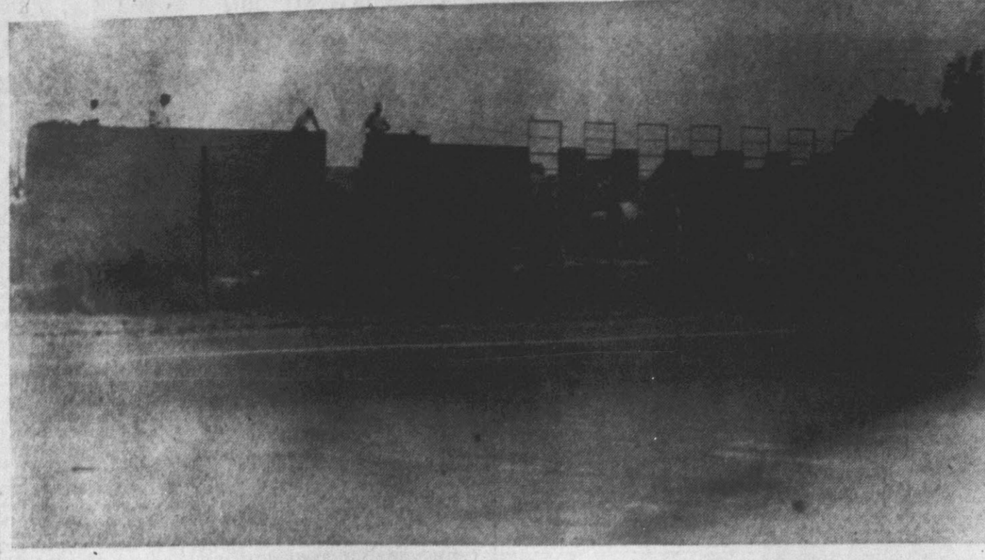
This view shows the new home of Greenville's Moose Lodge now under construction on the Farmville Highway across from the Raynor Warehouse. Upon completion the building will cover 11,000 square feet. According to reports the building, which will cost approximately $100,000, should be completed this fall. (Reflector Photo by Bob Boyette)
