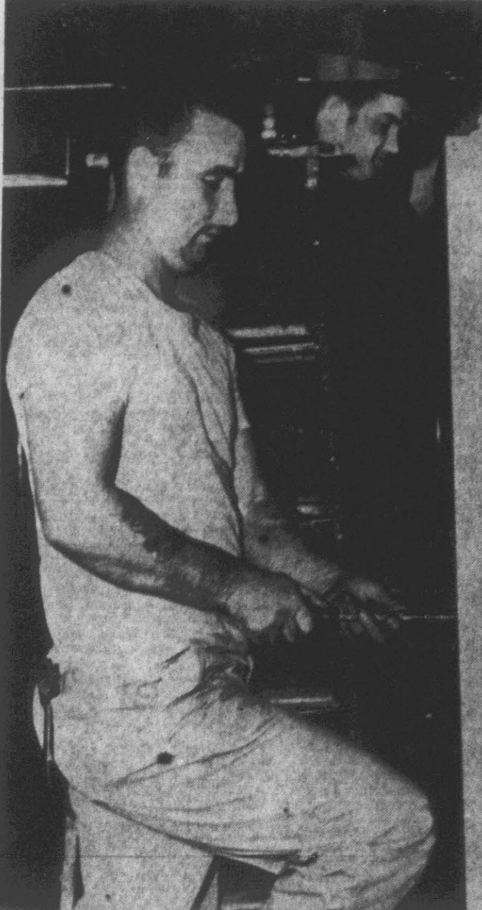
Workmen are shown above as they install the new air conditioning system in the police station portion of the municipal building. The system, which is to cost $10,437, is expected to be completed within the next few weeks. Sections of the building to be air conditioned include: the main lobby, the city manager's office, the downstairs portion of the police department, the Council room, and Greenville Utilities office. (Reflector Photo by Alvin Taylor)
