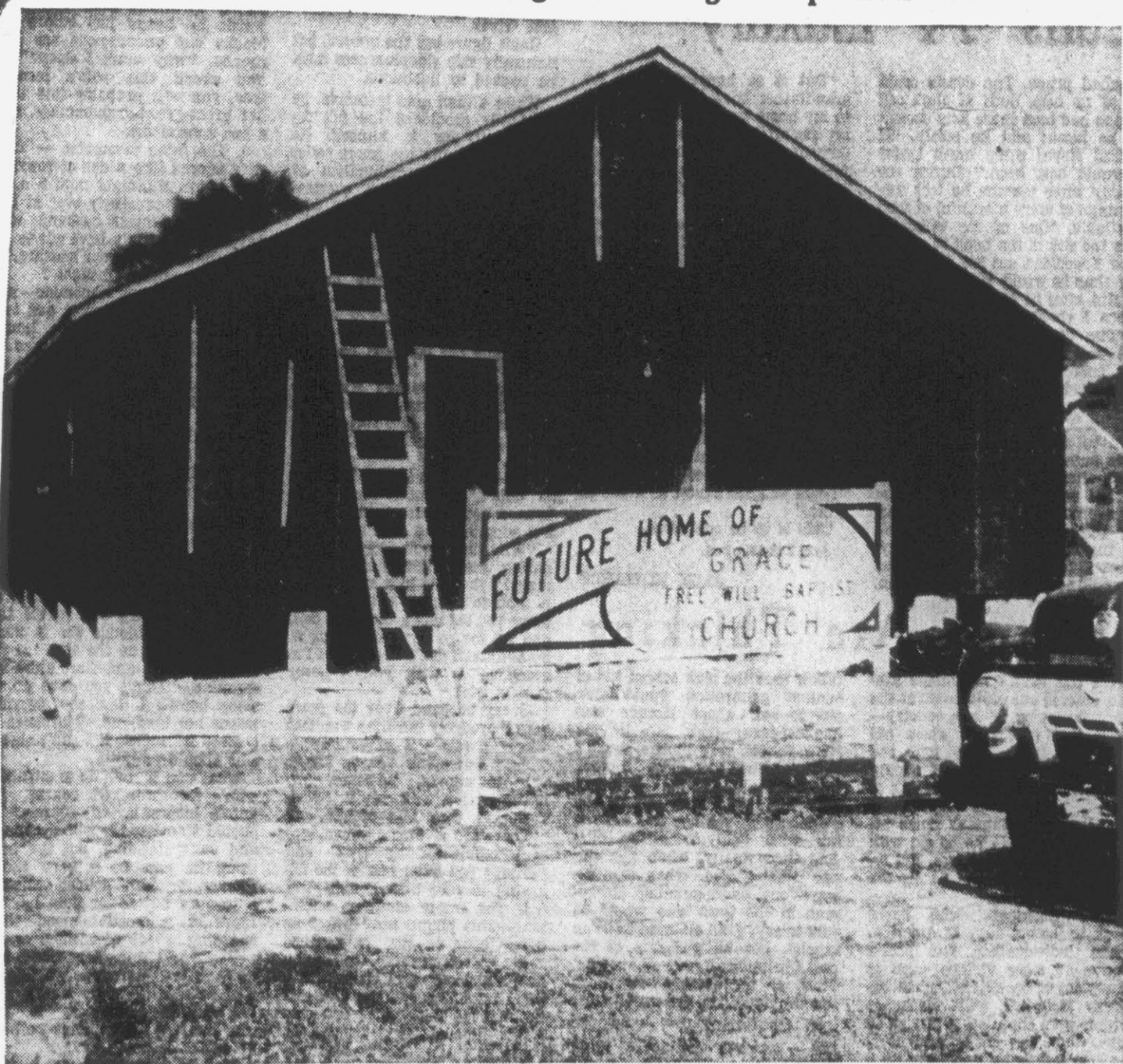
NEW CHURCH—Above is a view of the new Grace Free Will Baptist Church now under construction near the Village Grove section. The 40 by 100 foot building is the first unit of the church plant. It will serve as an educational building with space for worship, teaching and training. The Rev. Rashie Kennedy, pastor of the church, said that the interior of the building will be completed in time for a revival service to be held Monday night, May 24, and continuing through May 30. Rev. Kennedy said that the services will be held at 7:45 each night. When completed the building will be brick veneer and the pastor said that present plans call for moving all activities to the new church by June 1. (Reflector photo by Alvin Taylor)
