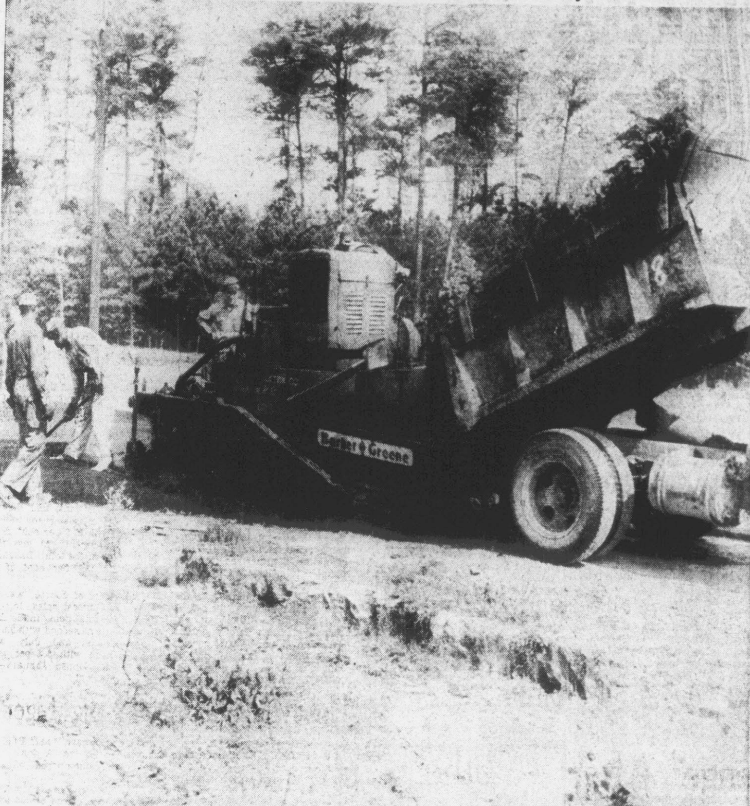
AYDEN STREET PROJECT—Workmen are shown as they work on paving one of the 11 blocks of streets in Ayden which are being surfaced. Workmen began yesterday morning on the paving project in Ayden, and according to Mayor Corey Stokes, are expected to finish the paving work by this afternoon. The town is paying one-third the cost of the paving, and the property owners the other two-thirds. (Reflector Staff Photo)
