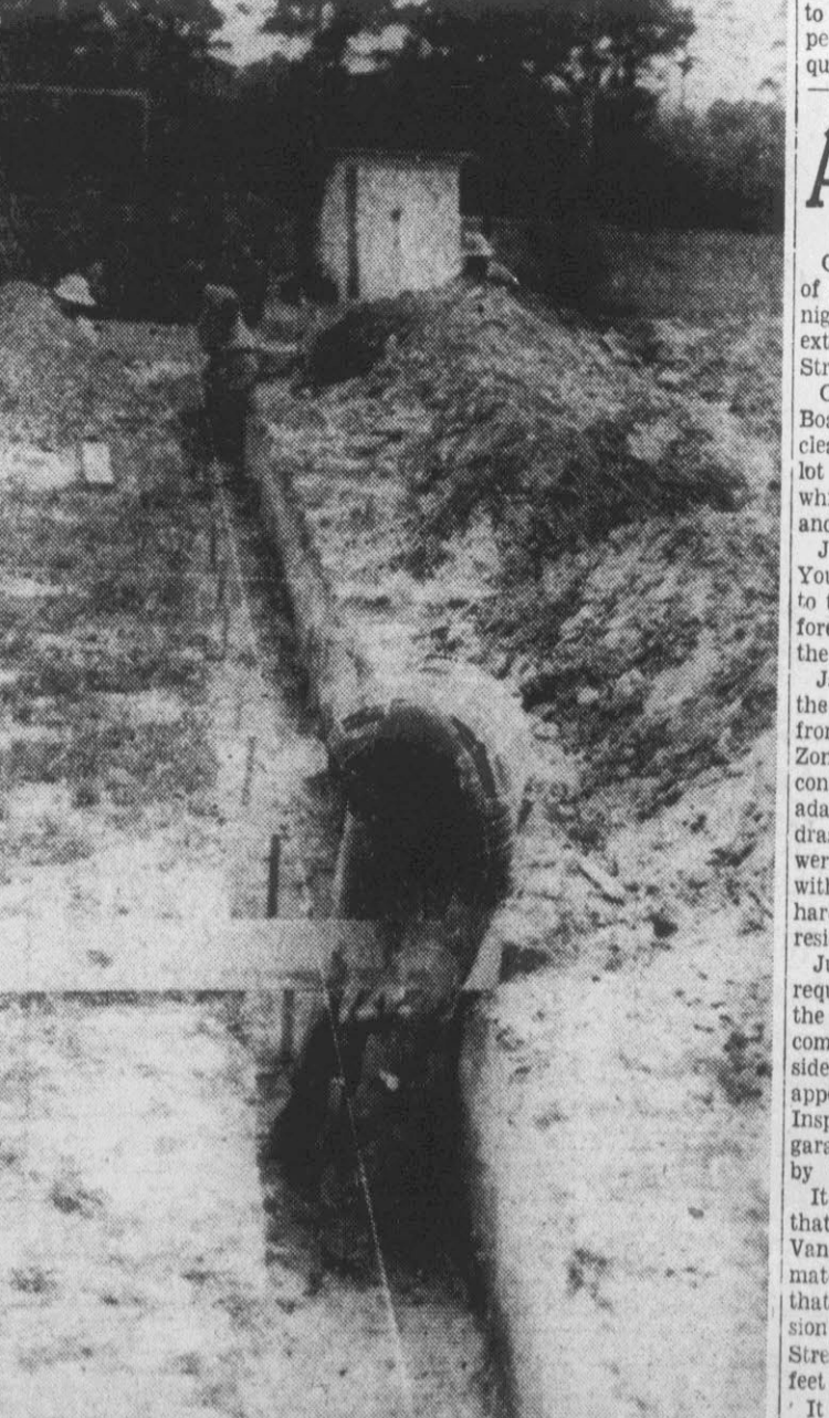
Workers are shown above as they prepare foundations for the new addition to South Greenville School. Under construction is the second wing of the building which will eventually be comprised of three wings. (Reflector photo by Alvin Taylor)
