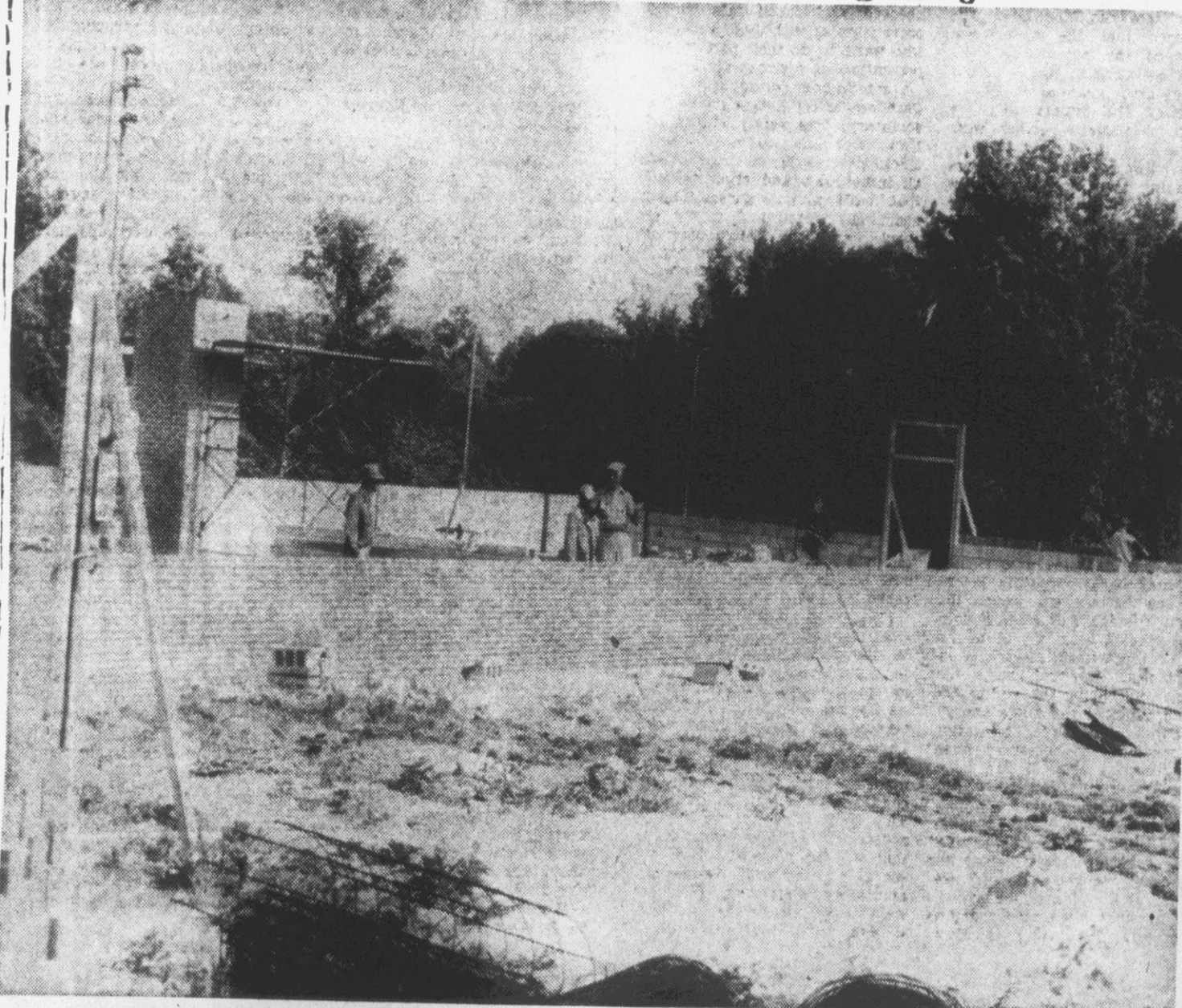
Work is progressing on the $100,000 St. James Methodist Church (above) now under construction in the Forest Circle section at East Sixth Street. Completion date has been tentatively set for November 1, according to the pastor of the church, J. Malloy Owen. The first section of the building will consist of a fellowship hall which will serve as a temporary sanctuary, an auditorium and a dining room. In addition the building will include a dozen classrooms, a kitchen and a pastor's study. Long range plans call for two additional sections to be added to the church. The St. James church now meets at Third Street School. (Reflector photo by Alvin Taylor)
