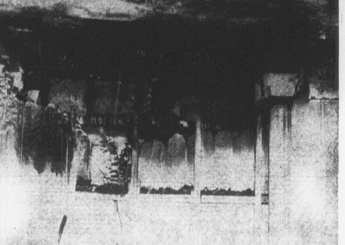
Pictured above is a view of the burned portion of a new home belonging to J. R. Moye. The above photo was taken in the den of the new dwelling. The fire, which started in a hall behind the den, burned completely through the wall separating the hall from the den. It also burned through the ceiling into the second story. Moye stated that the family had planned to move into the new home on April 10. He said that repairs will take from five to six months now, however. (Photo by Roy Hardee)
