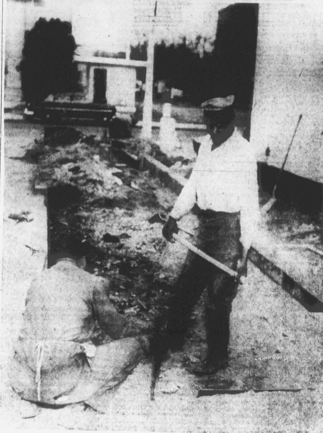
Workers are shown above as they break up the old curbing in the drive leading to the local post office. The drive is being widened to allow room for the large tractor-trailers now used in hauling the mail to enter. (Reflector photo by Alvin Taylor)
