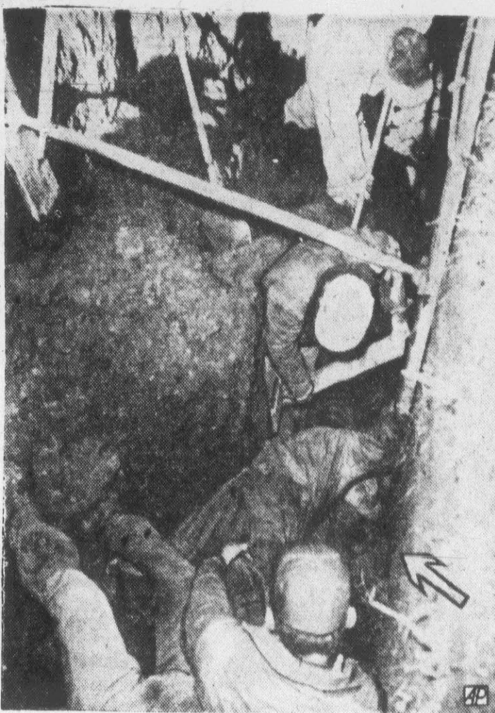
WORKER RESCUED —Fellow workmen work frantically to rescue Herman Koehn (arrow), 55, construction worker who was buried alive for more than an hour when a sewer trench caved in on him in Oklahoma City. One worker hung head down during the period to keep more dirt from falling on Koehn. Suffering only minor injuries, Koehn said he cupped his face in the bucket of the ditch digger to get enough air until his head was uncovered. (AP Wirephoto)
