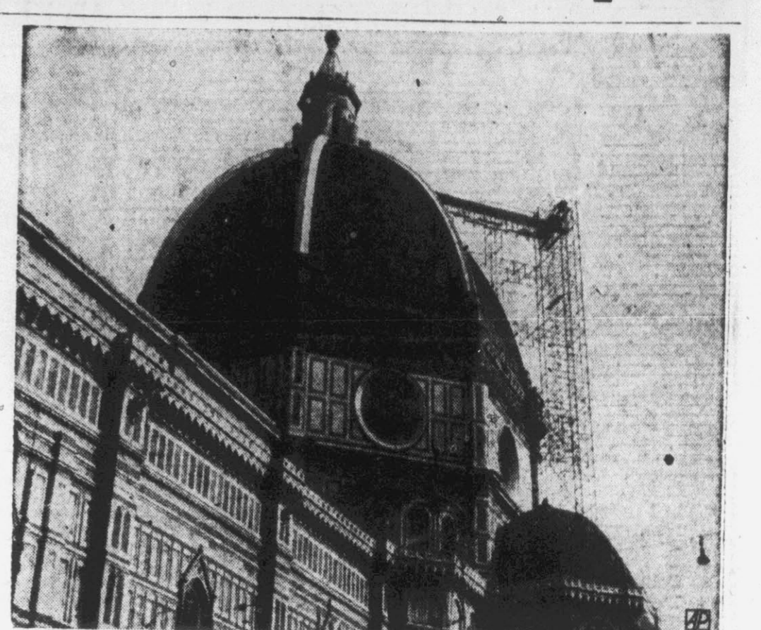
THE DUOMO GETS SHAMPOOED —The Duomo, Santa Maria del Fiore, world-famous Florentine church designed by Arnolfo di Cambio in the 13th century, is covered with scaffolding as workmen give its tiled roof a general overhauling to remove ravages of time.
