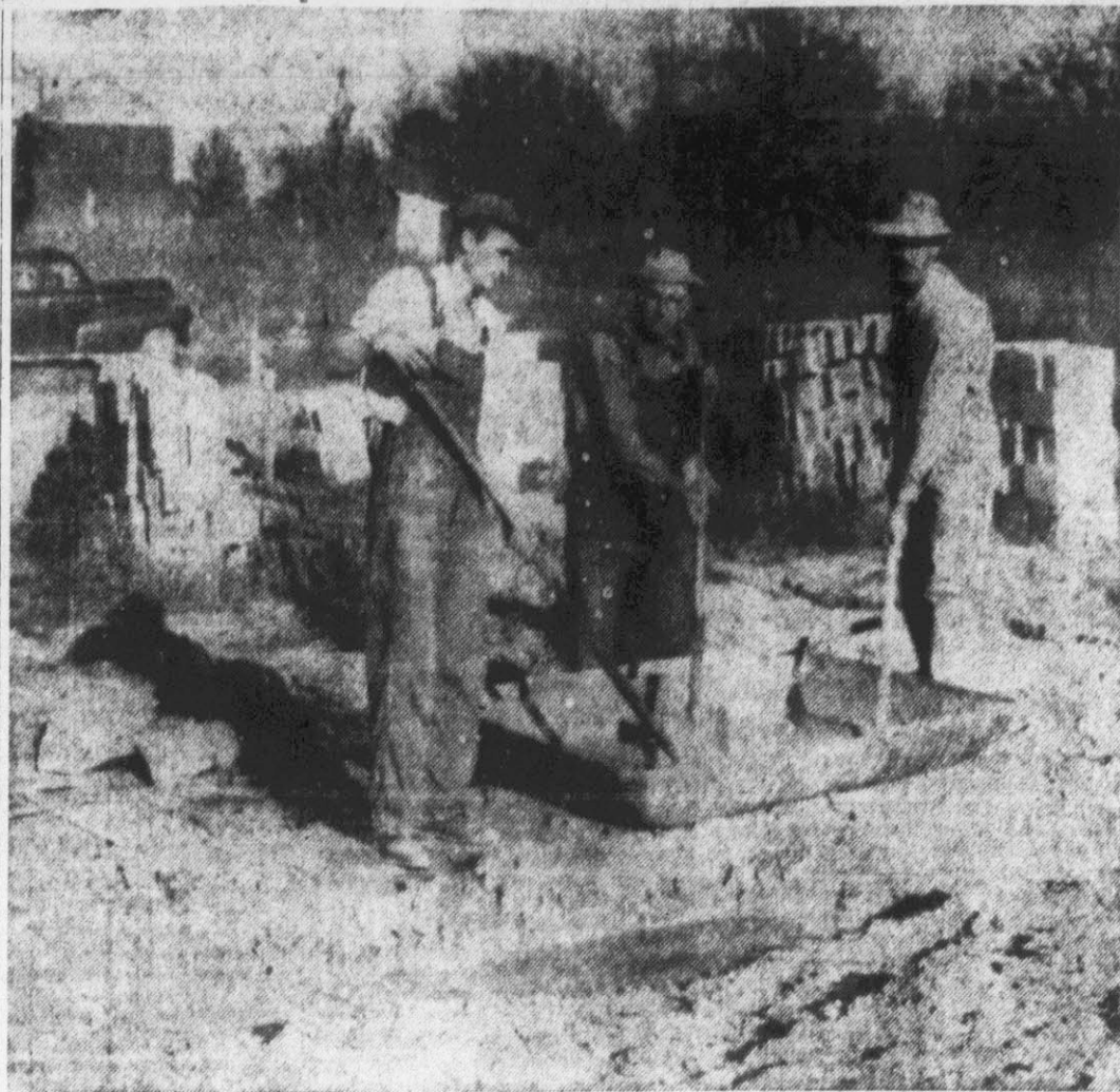
Pictured above are Marvin Stocks, E. B. Murphey and Robert Turnage as they lay the foundation for the new Free Will Baptist Church in Grifton.
