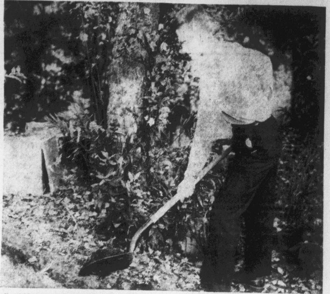
Jimmie Hendrix shovels dirt into the trench in which the irrigation system that he and his family are constructing at his home near Greenville is being installed. Hendrix is active in 4-H work and he won seven county championship awards this year.
