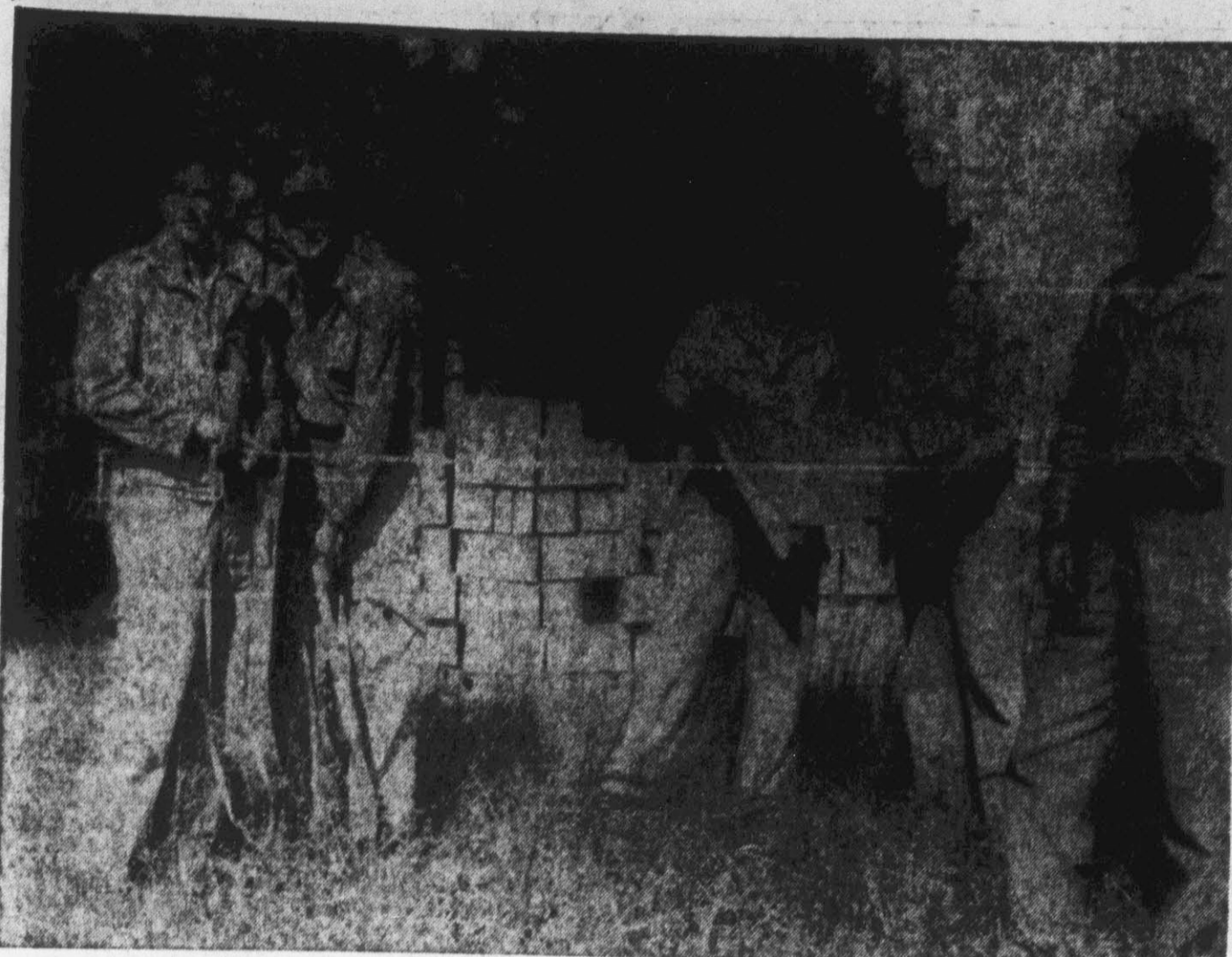
Members of the Falkland Ruritan Club begin work on the new Community Building for Falkland township. The building will have an assembly room 60 feet by 36 feet and a 11 by 25 foot kitchen. It is being built under the sponsorship of the Falkland Ruritan Club. Pictured above are Charlie Tyre, chairman of the building committee; Marvin Dean, treasurer of the Ruritan Club; G. A. Leonard; J. A. Moore; and Frank Corbett. (Reflector Photo by Alvin Taylor).
