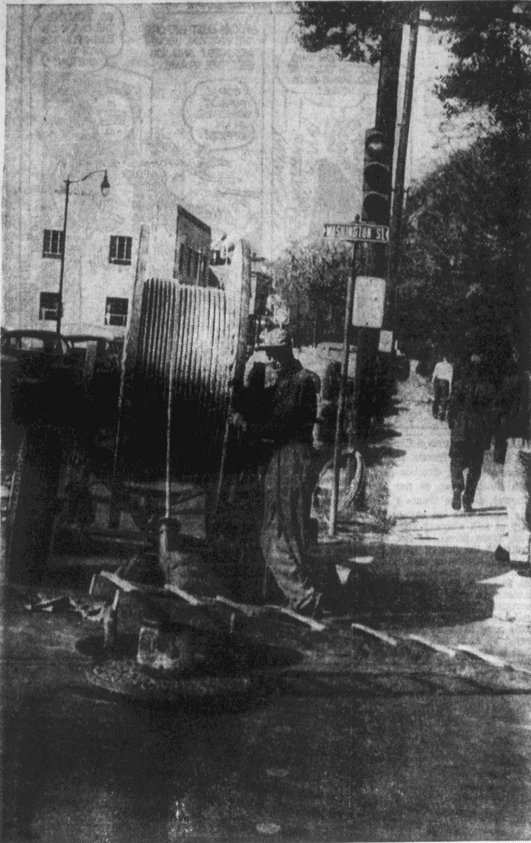
Telephone workers this week have been busy laying a portion of the coaxial cable over which network television shows will be brought into the Greenville area and Eastern North Carolina. The cable is being placed in trenches dug several weeks ago along Fifth and Evans Streets. (Reflector Photo by Roy Hardee).
