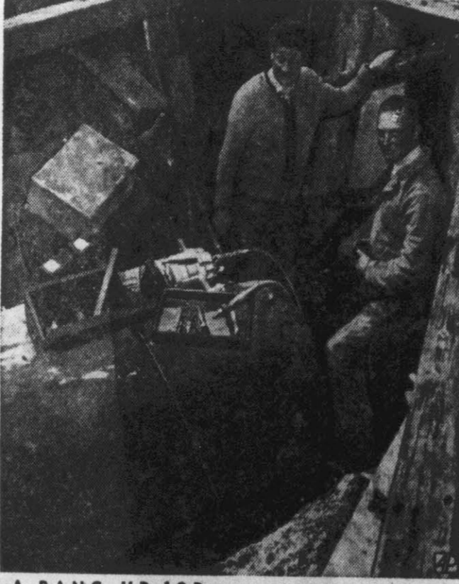
A BANG-UP JOB - Richard Hesse, left, and Erich Frodermann stand beside a two-ton blockbuster and they dismantled successfully in two hours near Neurnburg Castle, Germany.
