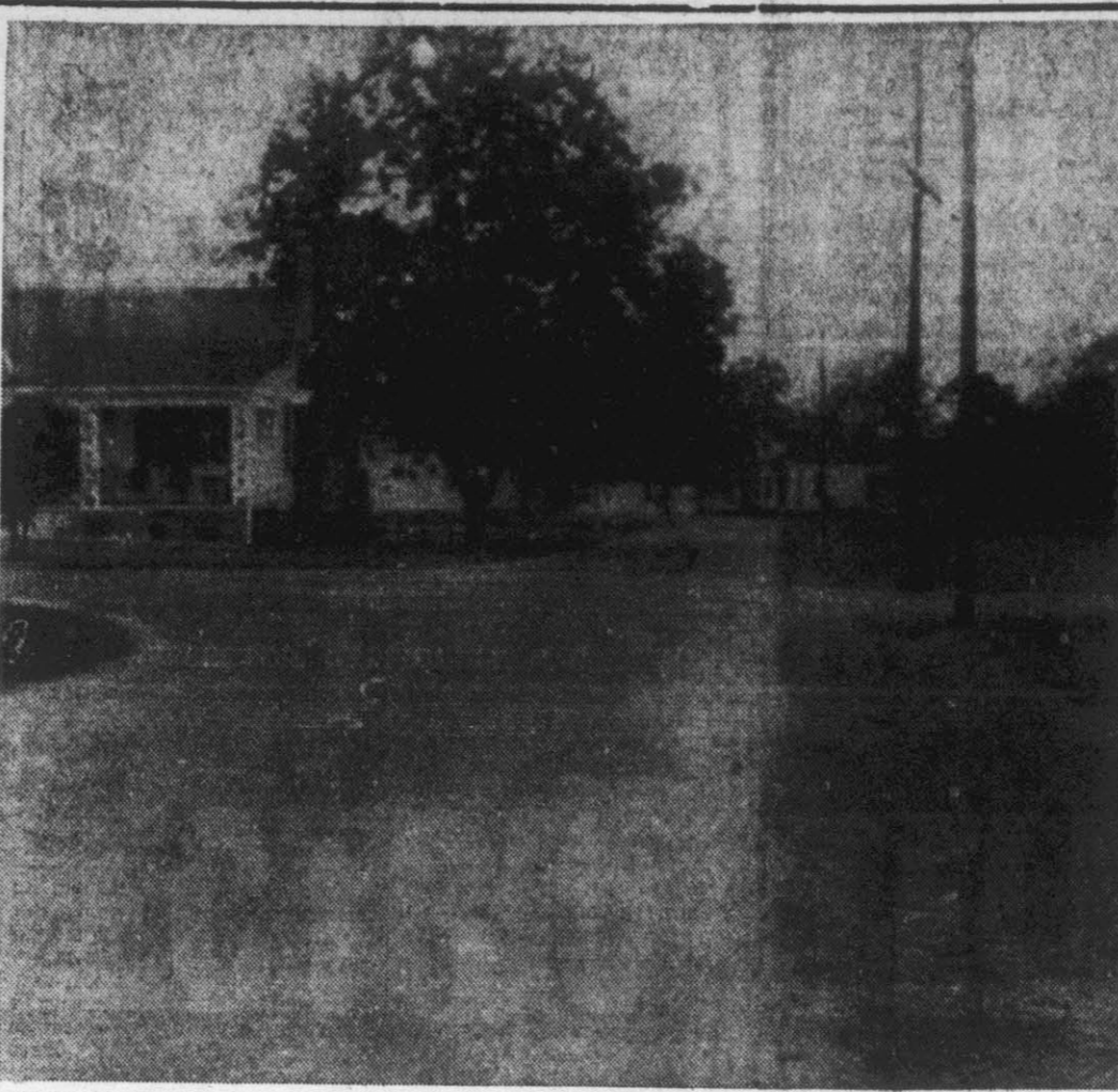
STREET WORK RECENTLY COMPLETED —The photo above shows a portion of street paving and street shoulder work in the Northeastern section of Greenville recently completed under the supervision of the Street Department. Paving on approximately eight blocks of A Street, B Street, Jarvis Street and Summit Street were recently completed as property owners paid cash for 100 per cent of the cost of paving. The Street Department yesterday completed work on the shoulders of the streets, grading them, and planting grass seed. (Reflector Staff Photo)
