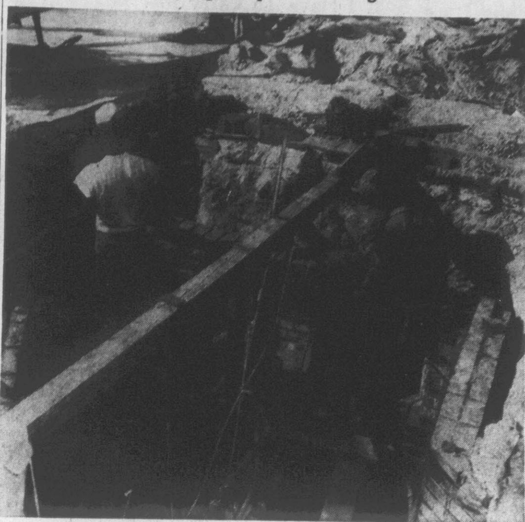
That big hole in the middle of the street at the intersection of Fifth and Washington, which has obstructed traffic for several days, is just another part of the laying of the TV cable which will bring network programs to Eastern North Carolina when the local station goes on the air. (Reflector Photo by Roy Hardee)
