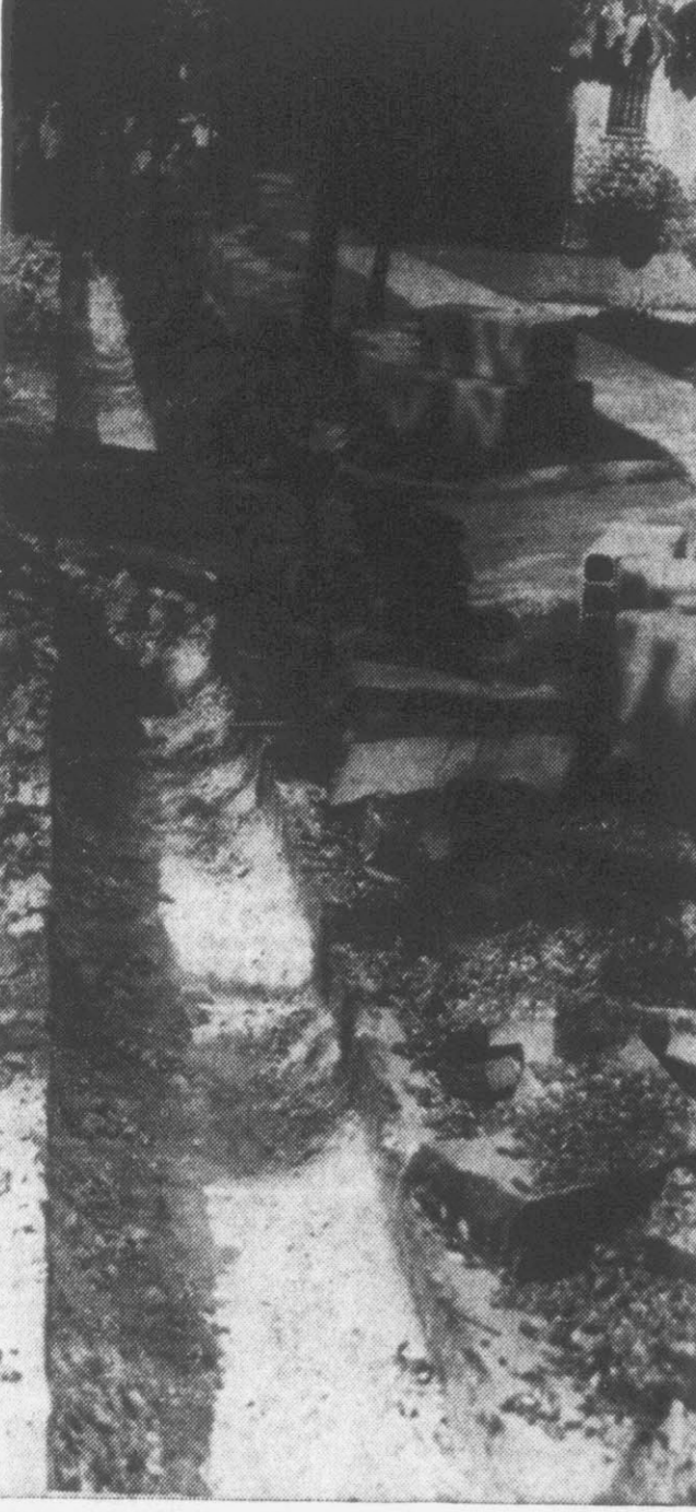
Work on the television cable which will bring network shows to Greenville's TV station, is moving along. At the present time, construction work has passed the intersection of 12th and Evans Streets, extending toward the station. In the uptown business section, work on resurfacing streets turn up to lay the cable, was begun yesterday. (Reflector Photo by Roy Hardee)
