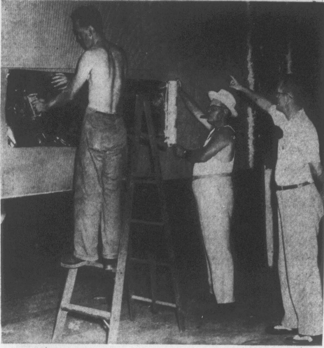
Preparations for next week's Farmers' Day are well under way at the New Enterprise Warehouse, scene of this year's celebration. Shown above directing work on a partially completed stage in the warehouse are, center, professional decorator Jack Finch, and right, Farmers' Day Steering Committee Chairman Jack Wallace. Finch, a veteran of 35 years in the decoration field, has done the Farmers' Day here since its inception 5 years ago. On the ladder with the staple gun is Burt Moore of Boone, a member of Finch's crew. (Reflector Photo by Al Perry)
