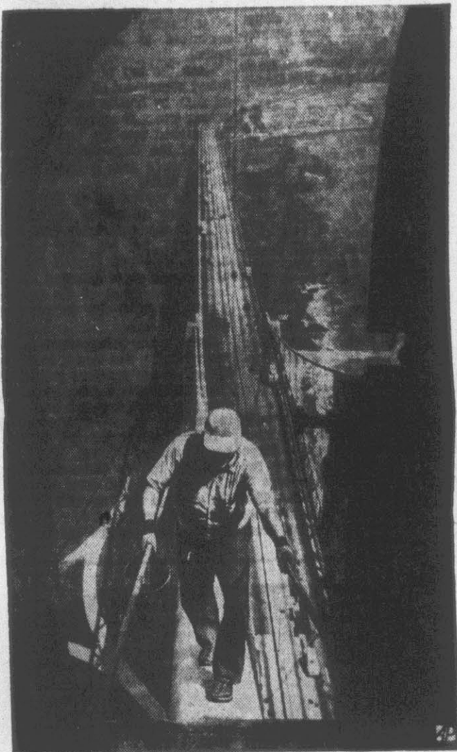
STEPPING HIGH —A painter, climbing to top of one of two 363-foot towers of New York's Bronx-Whitestone Bridge, is member of crew giving span its first paint job in six years.
