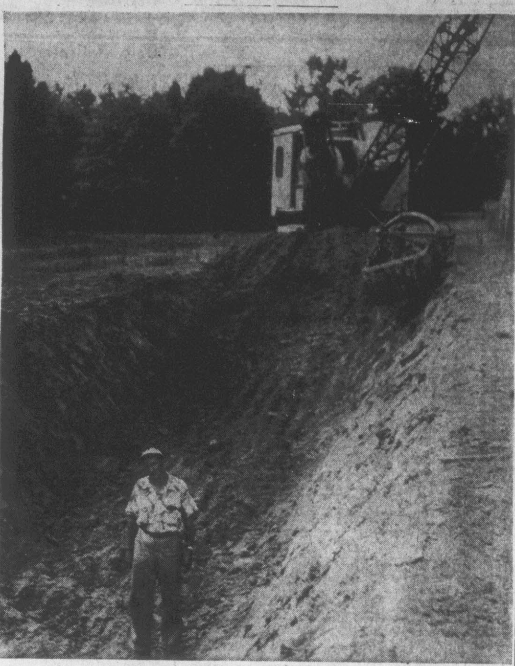
SILGO GOES UNDERGROUND —Bill McLawhorn glances up from and inspection of work going forward on his new "underground" silo in which the Pitt county farmer hopes to store several acres of corn soon. The corn will be cut soon after it is mature and packed into the nine-ft. deep trench. Then it will be packed tight and covered with tar paper and packed layers of sawdust. By winter he hopes to have plenty of good silage to assure his cattle of ample "vittles." He is being assisted in the project, first of its kind in this county, by Conner Eagles, United States soil conservationist for this area. The silo is on the McLawhorn farm near Ayden. (Reflector Staff Photo)
