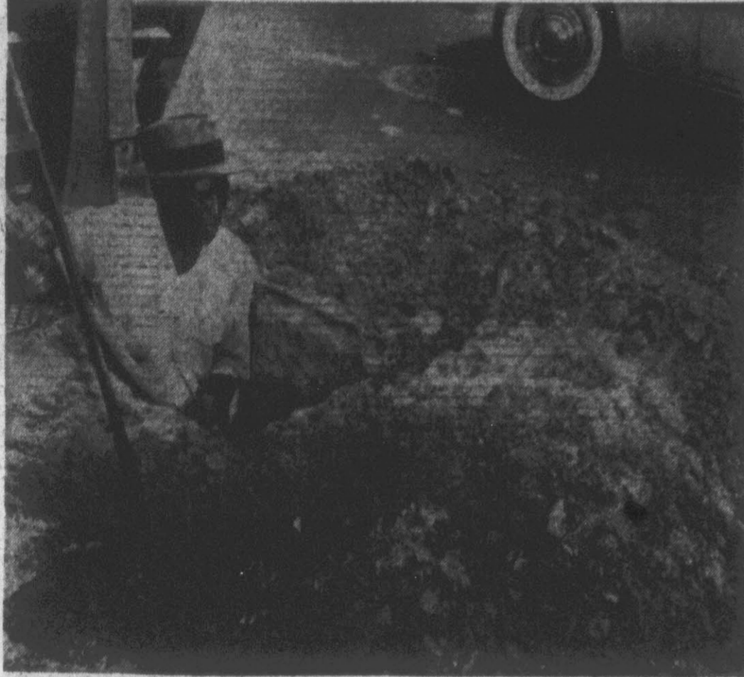
In preparation for installing a new type of illumination for Evans Street, a Greenville Utilities working crew has been engaged in readying foundations for new light poles. The aluminum poles will suspend the lights approximately 21 feet above the street. (Reflector Photo by Roy Hardee).
