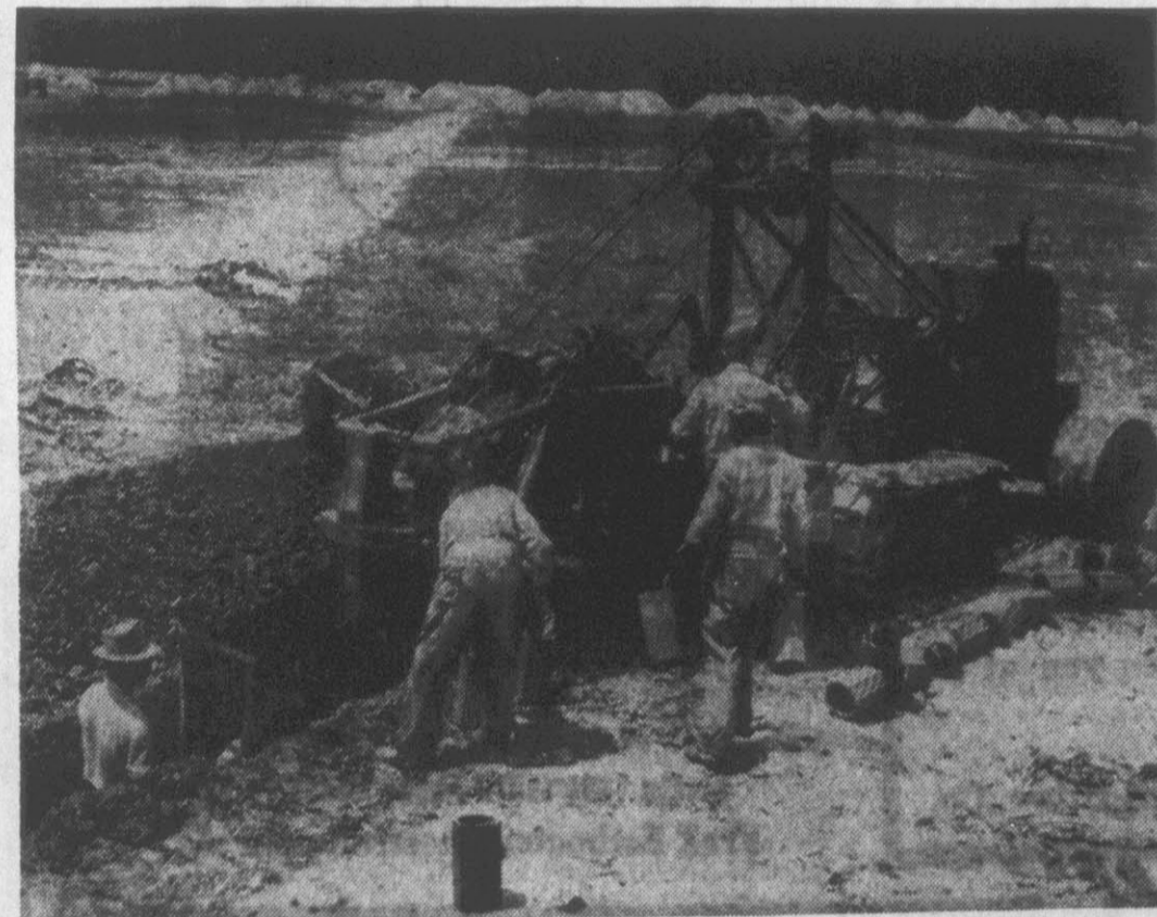
WET LAND INTO DRY —Last year county farmers placed nearly 150,000 additional feet of drainage tile into use on their farms. Shown above are workers installing field tile which will enable the wet and unserviceable land to be drained and placed in active production of many farm crops. (Reflector Photo by Roy Hardee)
