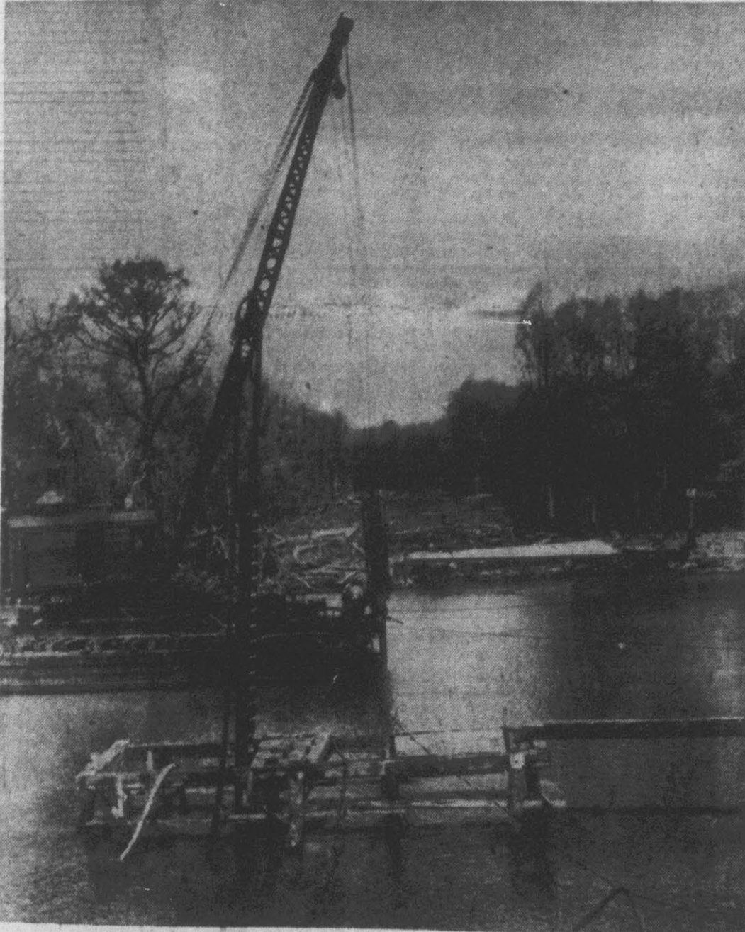
NEW BRIDGE FOR GRIMESLAND - Work on a new bridge across the Tar River at Grimesland started recently to replace the old bridge which has been declared a hazard. Piling are being driven into the river bed, as shown in the picture above. (Reflector Photo by Roy Hardee)
