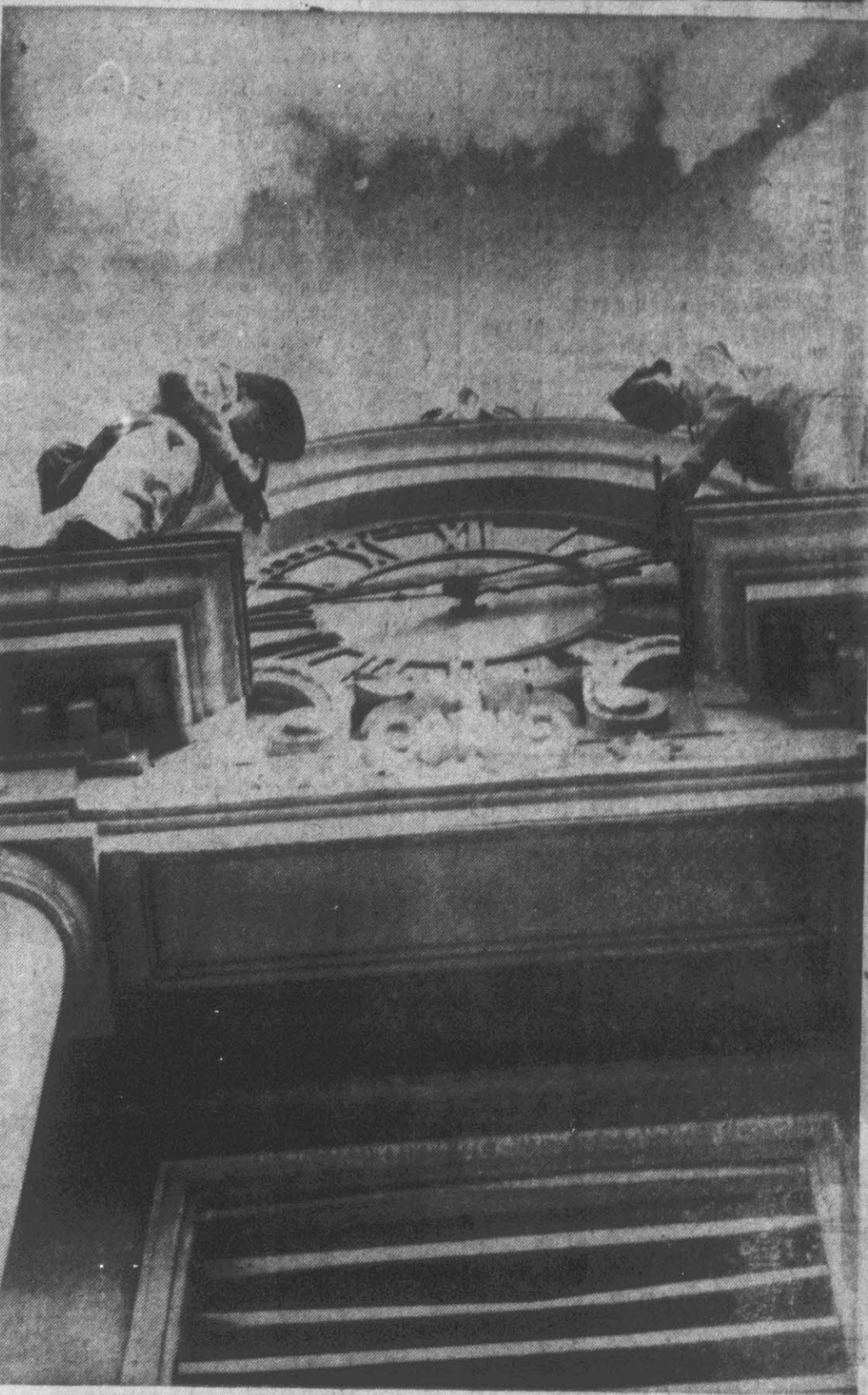
ANYBODY GOT THE TIME? Yes, it's a quarter to three by the courthouse clock. The two high-altitude painters shown above will testify to that, because they are re-finishing the face of the county timepiece. That's "Al" by the minute hand to the left, and "Chuck" is directly to the right of the hour hand.
