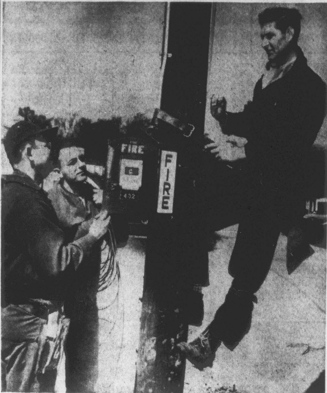
Enlargement of Greenville's present fire alarm system was partly completed yesterday when seven new alarm boxes were installed. Delayed for nearly two years, due to a shortage of copper wire, the project calls for the erection of 14 new call boxes in various sections of Greenville now isolated from the fire alarm network. Most of the boxes will be placed in new subdivisions which have been built after the present system had been installed. Above, firemen Alton Vincent, Claude Christopher, and Ray Smith are shown placing box 432 in operation. This box is located at Liberty and Willow Streets. (Reflector Photo by Roy Hardee)
