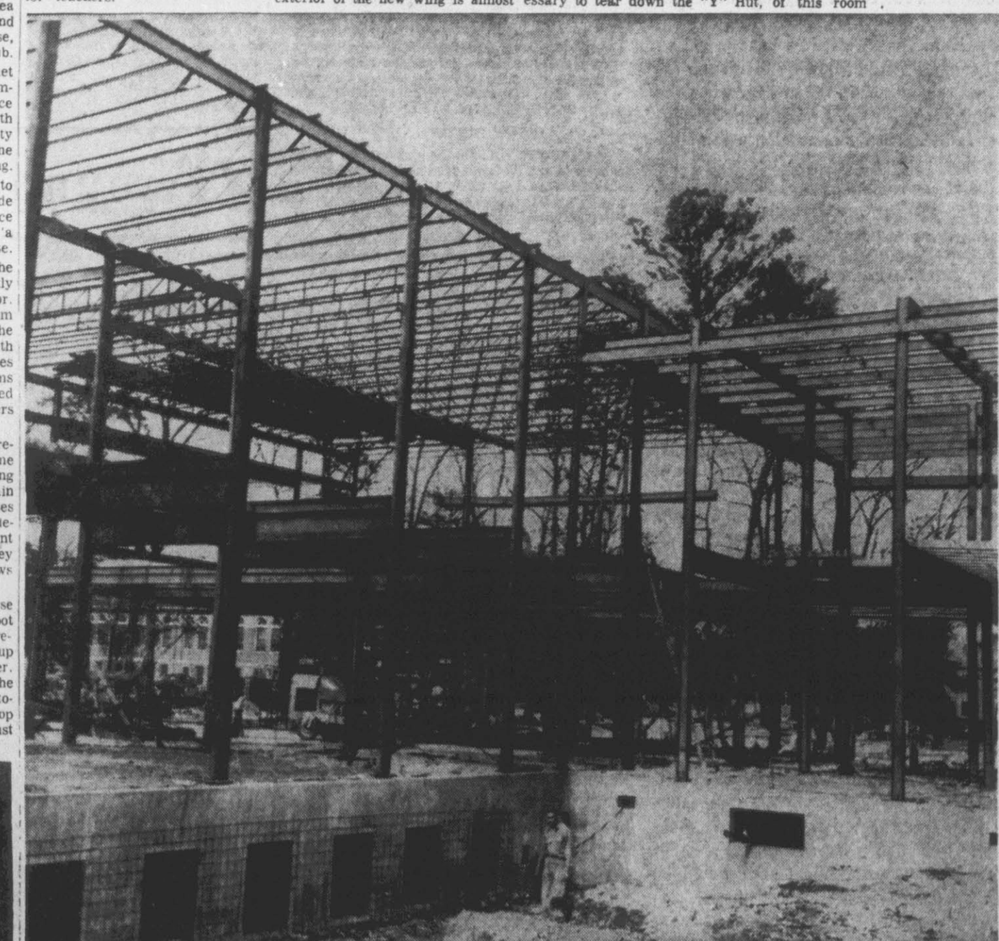
JOYNER LIBRARY. Named for a noted North Carolina educator and former State Superintendent of Public Instruction, Dr. J. Y. Joyner, the new library at East Carolina College is rapidly taking shape. The structure will contain stacks for a collection of 117,000 books, in addition to classrooms, projection room and broadcasting studio.
