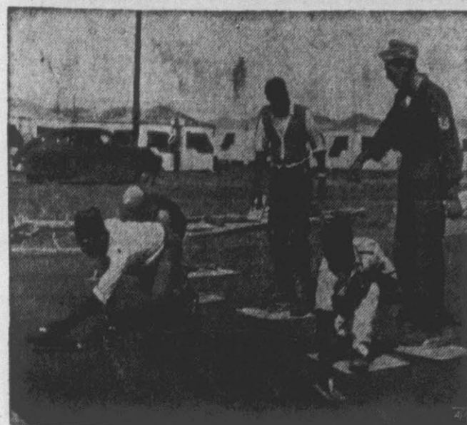
MOROCCANS lay concrete tennis court at Sidi Slimane, U. S. Army Base. T-Sgt. Richard J. Leapley of Sioux City, a., directs work paid for without congressional aid.
