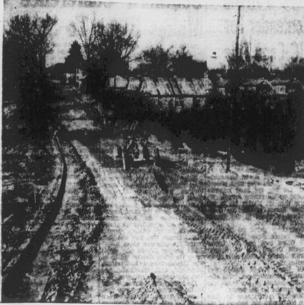
The grading of Second Street, from Cotanche through the "valley" to Jarvis Street is almost complete. The Greenville Utilities Commission has completed installation of its facilities and 98 per cent of the curb and guttering has been installed. Asphalt paving will be laid until the earth settles... which process may require as long as 90 days. (Reflector Photo by C. L. Perkins Jr.)
