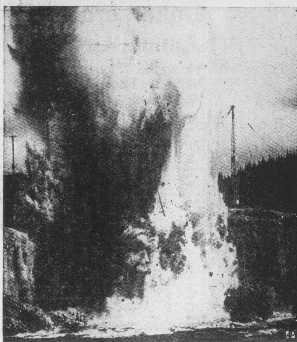
CONVERTING NATURE TO MAN'S SERVICE — Water and rocks hurtle skyward from Waikato River in New Zealand as stream is diverted to make room for power station.
