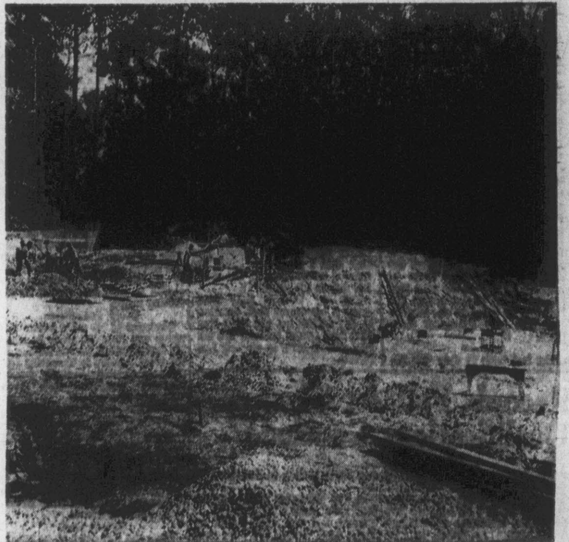
Construction work on the new Joyner library at East Carolina is moving briskly ahead.
