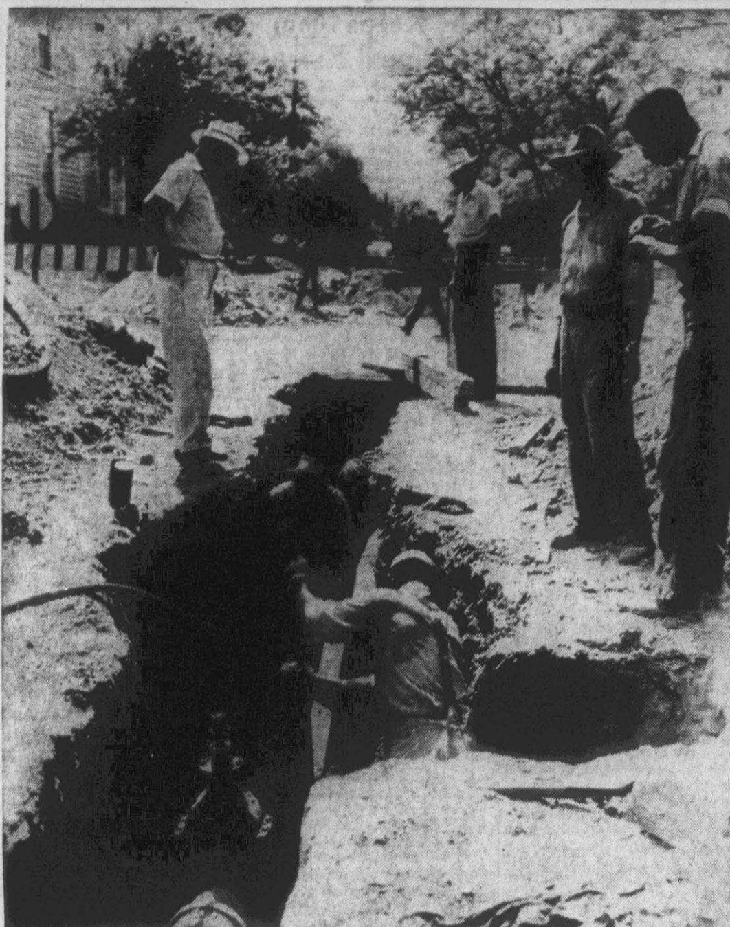
Employees of Greenville Utilities Commission are shown making preparations to connect the six-inch water line that serves North Greenville with the new 12-inch main from the Water Plant. The above excavation at the corner of First and Greene streets is the point where the two lines converge, and the tie-in is calculated to raise the pressure across Tar River—thus providing more efficient service and increasing fire protection. Supervising operations are (left) Elmo Savage, in charge of heavy construction, and gang foreman Mack Fleming.—(Photo by C. L. Perkins, Jr.)
