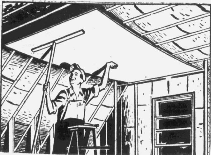
ONE MAN can install gypsum wallboard panels on attic ceiling by using a T-brace to hold end of the material. Notice insulation shown between rafters and ceiling joists.
