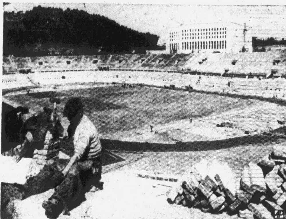
SOON TO BE COMPLETED — Work is rushed on Rome's Olympic Stadium so it can be finished for the England-Italy soccer match in May. Stadium will hold 81,000 spectators.
