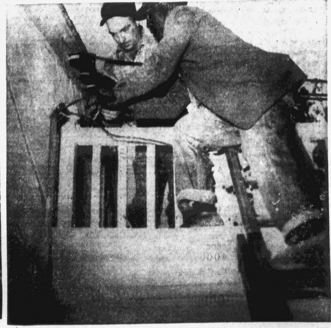
The final step in bringing power into a rural home is made by two workers when they connect the lead in power lines to the household wiring as shown above.
