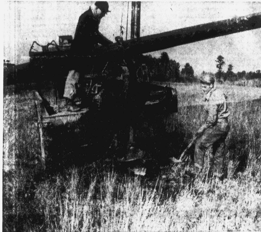
This labor saving machine, a boring instrument, can dig a hole to place a pole in less than two minutes. Then the hoist swings the pole around and drops it into the freshly dug hole.
