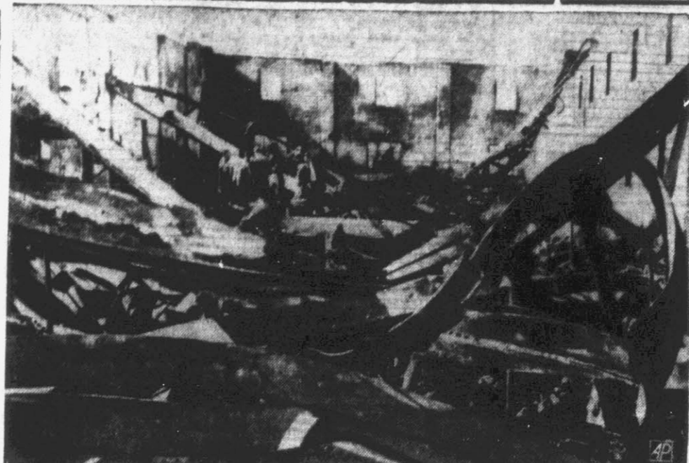
TWISTED RUINS AFTER CHRISTMAS PARTY.—Steel girders lie twisted between concrete walls where at least 41 persons, mostly women and children, perished in a Christmas party at Tijuana, Mexico. The party was on the top, third floor (shown here) and the only exit was down stairs through a single door. Eighty-eight others of the crowd of from 300 to 400 at the party were burned or injured, 32 seriously. (AP Wirephoto)
